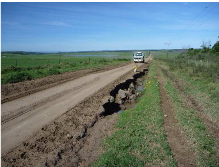
Figure 33 Erosion due to erodible materials and human activities
