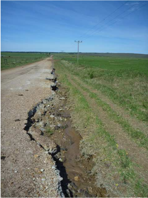
Figure 34 Erosion due to erodible materials and human activities
