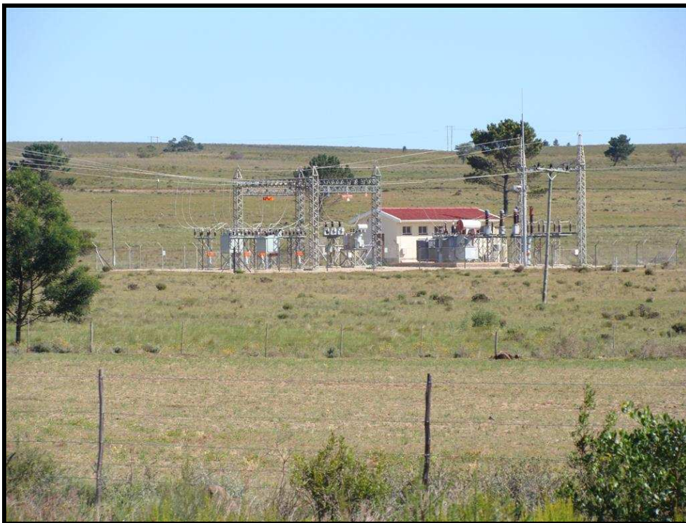
Photograph 1.1: Existing Dieprivier substation on farm Dieprivier.
