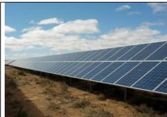
Figure 2.2: Picture of a PV Panel Modules (75 MW plant in Kalkbutt South-Africa Source: SMA)
