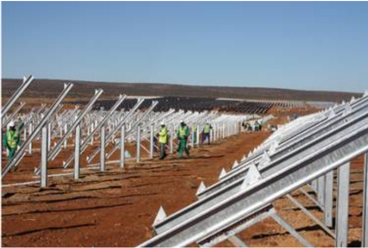
Figure 2.7: Frame, structural details (Lesedi Solar PV Project, Kimberly, South Africa. Source: Power Technology.com).
