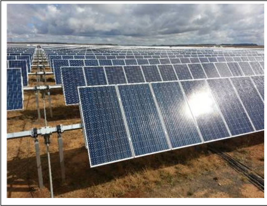
Figure 2.6: The support structures elevate the PV panels and allow for single axis tracking of the sun for increased efficiency (Source:SAPVIA)
