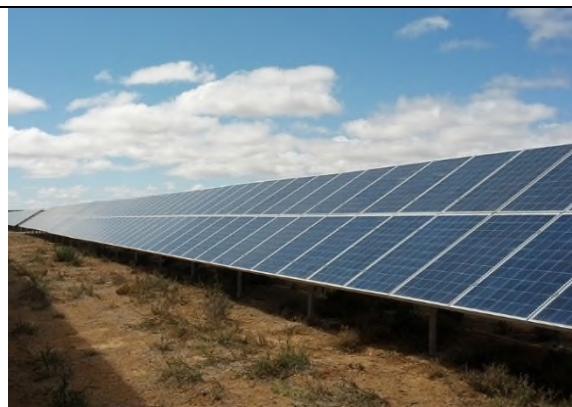
Figure 2.4: Picture of a PV Modules (75 MW plant in Kalkbutt South-Africa Source: SMA)
