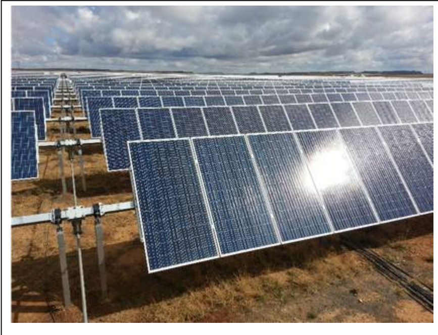
Figure 2.6: The support structures elevate the PV panels and allow for single axis tracking of the sun for increased efficiency (Source:SAPVIA)
