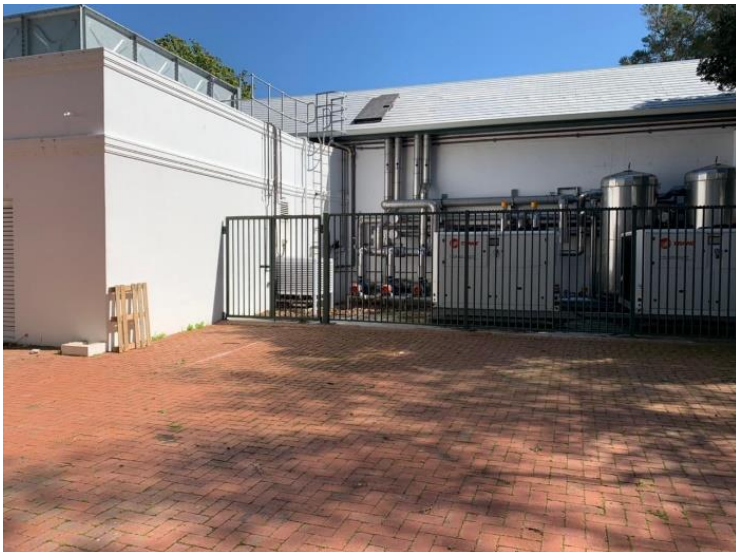
Figure 5: Shows the Mechanical Plant
