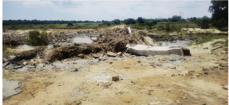
Photo 2: Damaged bridge on S722 Road
