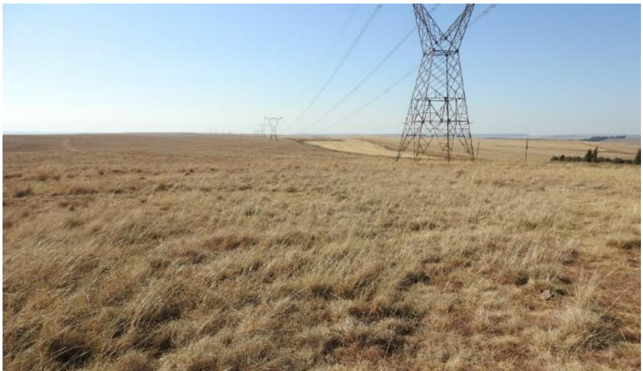
Figure 5: High voltage lines
