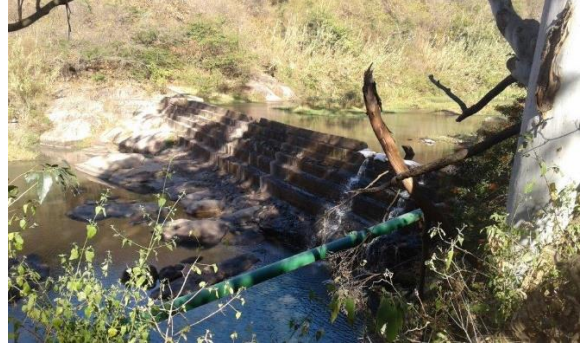
Photo 4: View from the left hand bank of the Umzinto River looking from north to south across the river showing the proposed site of the new gauging weir which will be mounted on the existing infrastructure.
