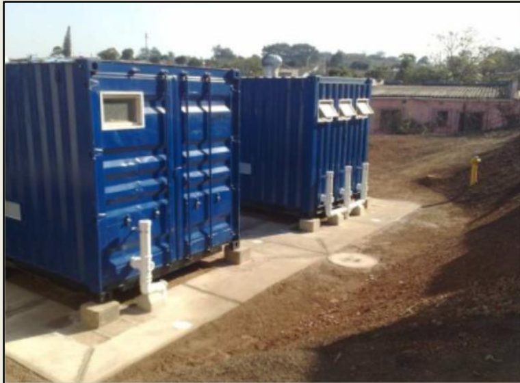
Figure one: Prefabricated container and associated pipework (Source: eThekweni Water and Sanitation, 2010)
