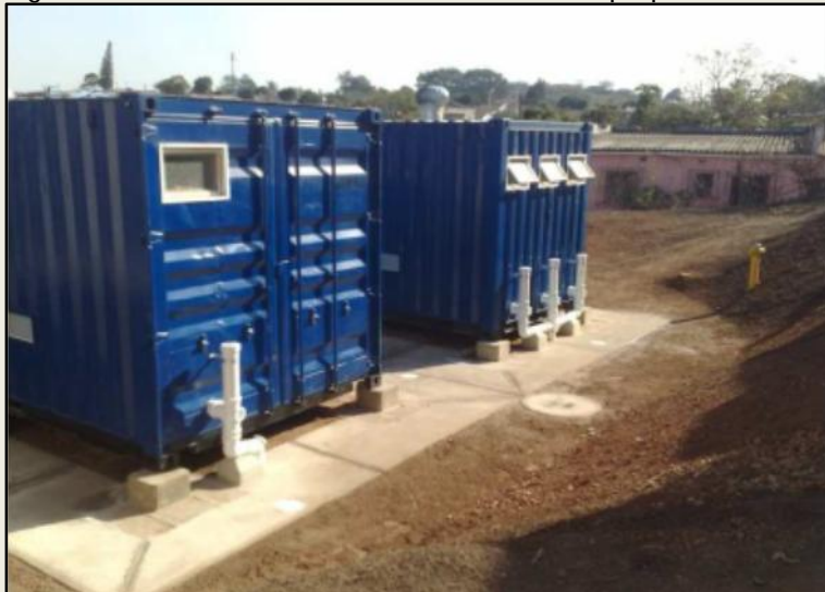
Figure two: Prefabricated container in Durban (Source: eThekweni Water and Sanitation, 2010)
