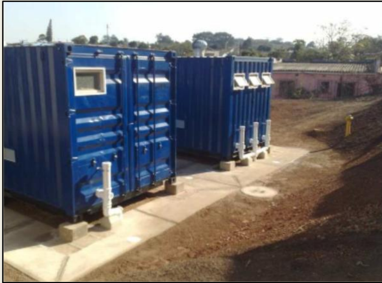
Figure one: Prefabricated container in Durban (Source: eThekweni Water and Sanitation, 2010)
