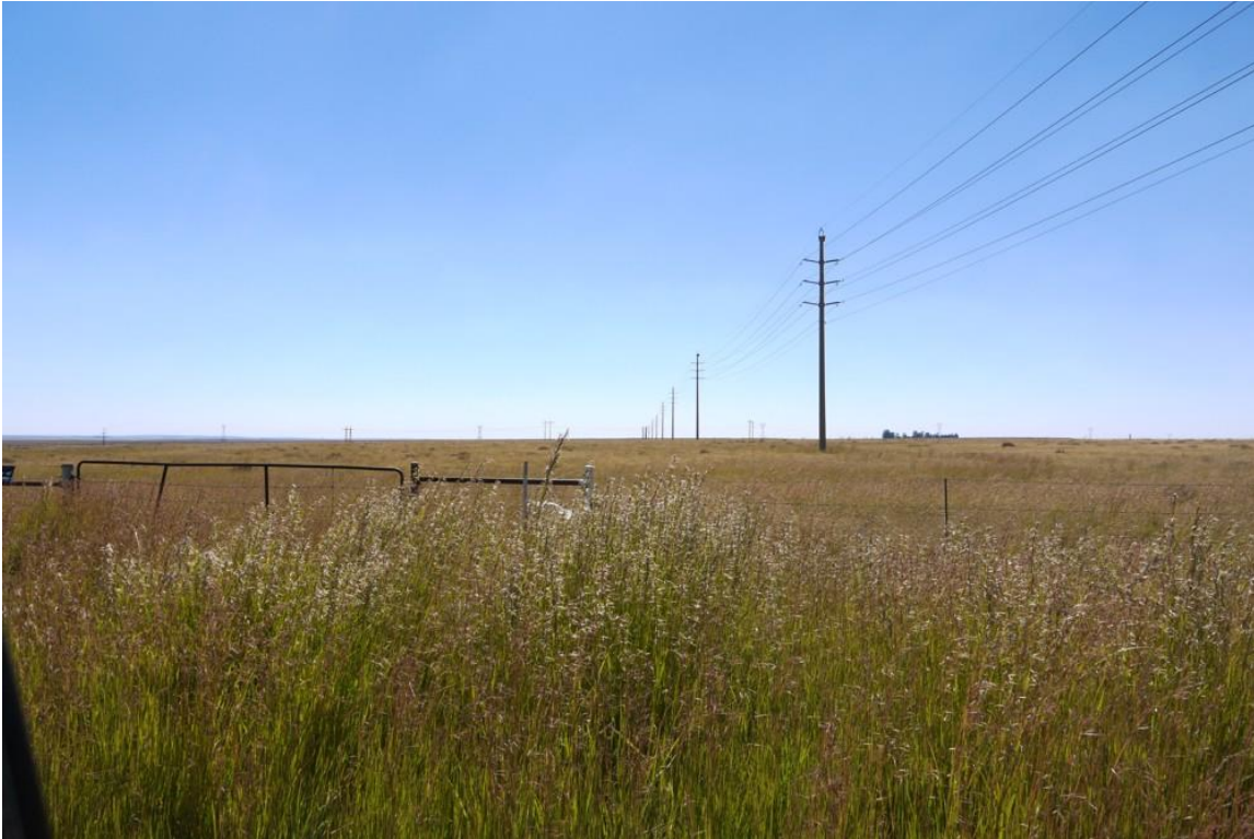
Plate 8, A view along the line of a 132kV overhead power line with monopole towers
