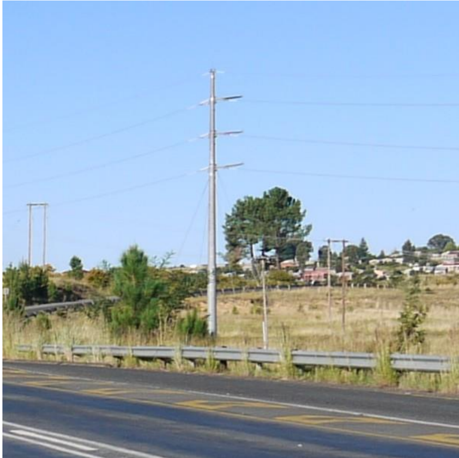
Plate 3, Typical 30m high 132kV self-sustaining steel monopole tower
