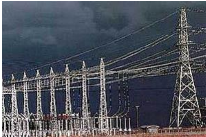
Plate 1, Transmission lines leaving an MTS.
