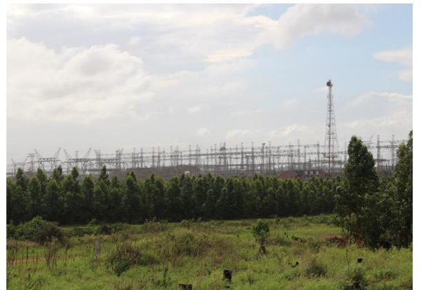
Plate 18 - Sub-station & Communication Tower
