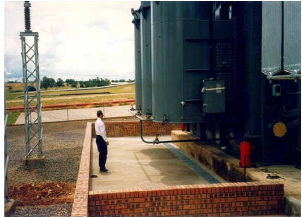
Plate 16 – Transformer approximate height 10m
