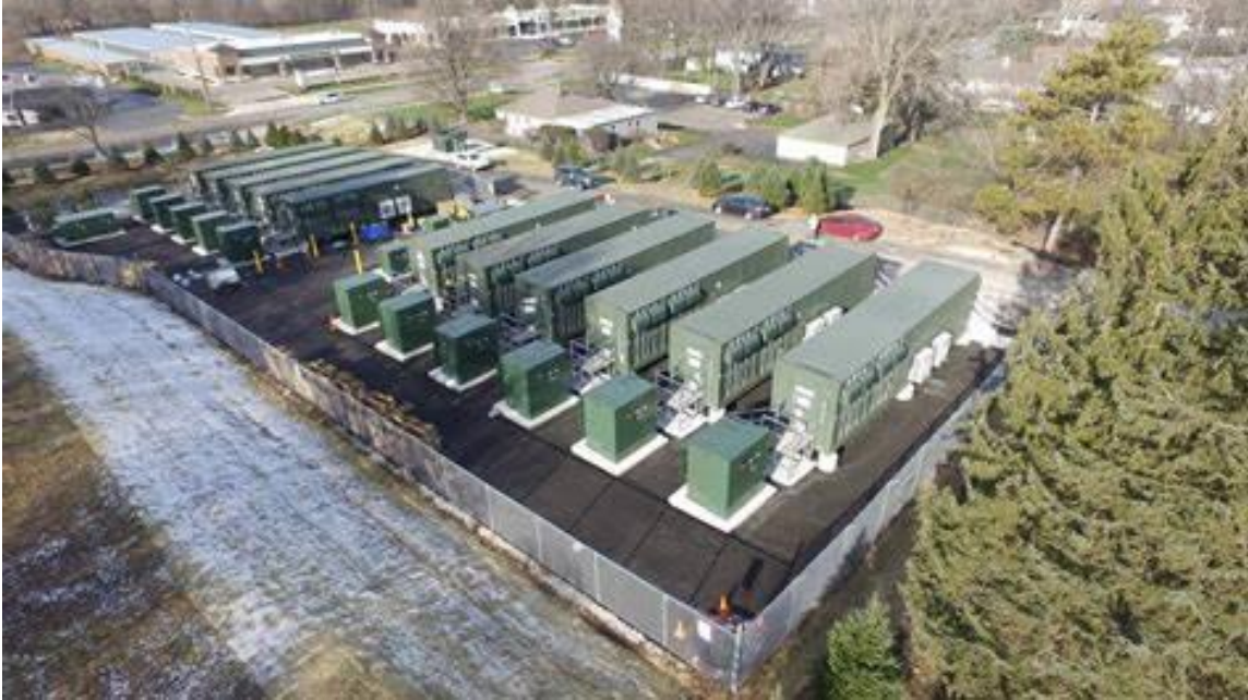
PLATE 2 TYPICAL BATTERY ENERGY STORAGE SYSTEM
