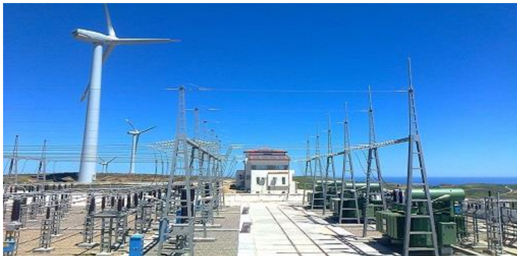
PLATE 1, BUS BARS ARE THE HIGHEST SUBSTATION ELEMENTS IN PICTURE
