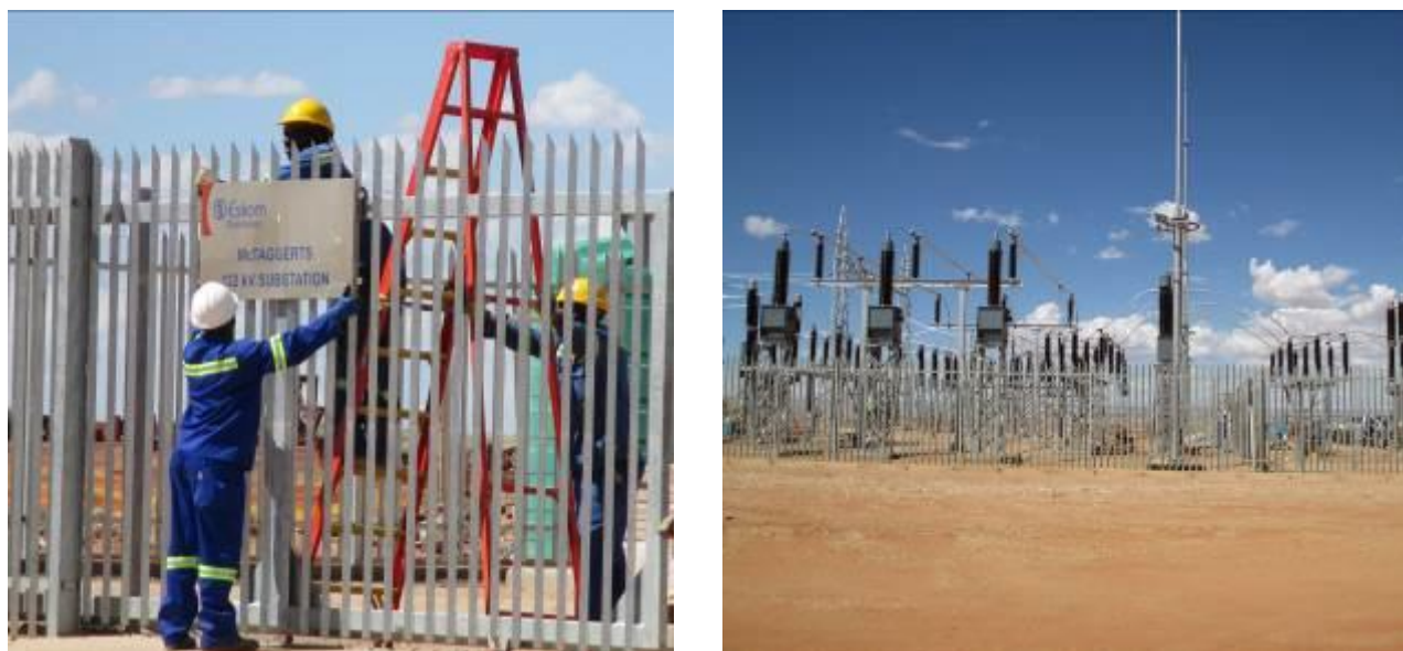
Figure 3.5: Photographs of the newly constructed McTaggerts Substation located on Portion 3 of the farm McTaggarts Camp 453
