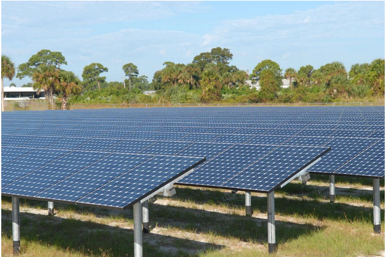
Figure 2-4: Photovoltaic (fixed-tilt/ static) panel array
