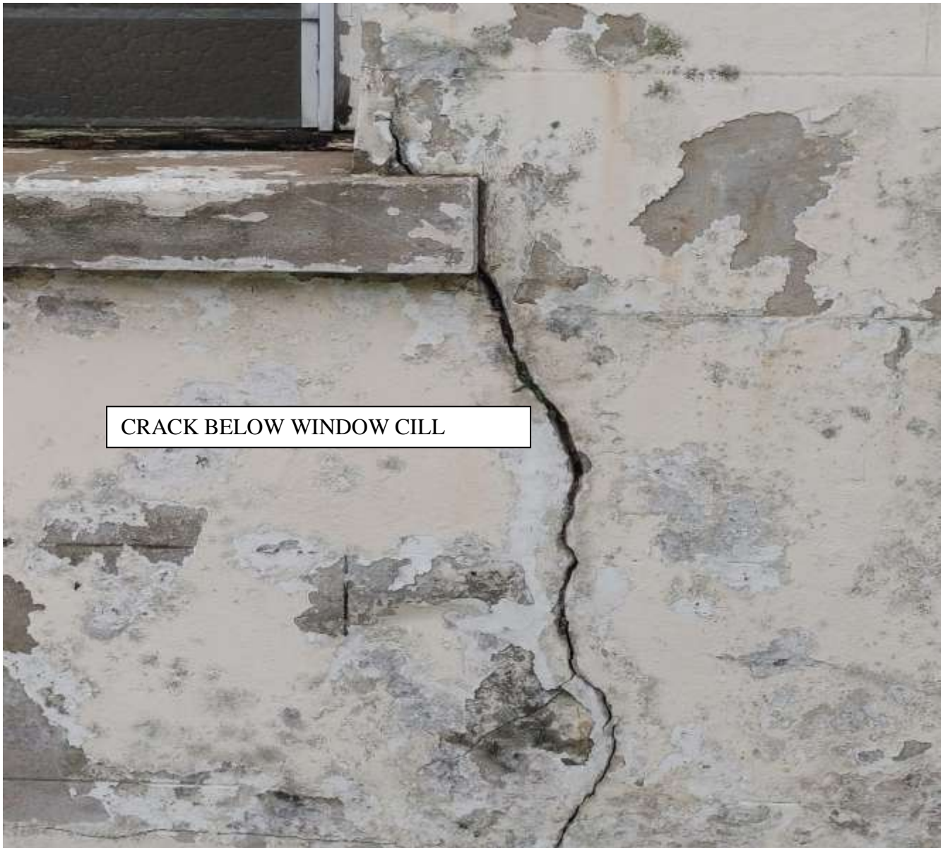
FIGURE 3 : SETTLEMENT OF FOUNDATIONS / CRACKS AT CNR OF WINDOW CILL
