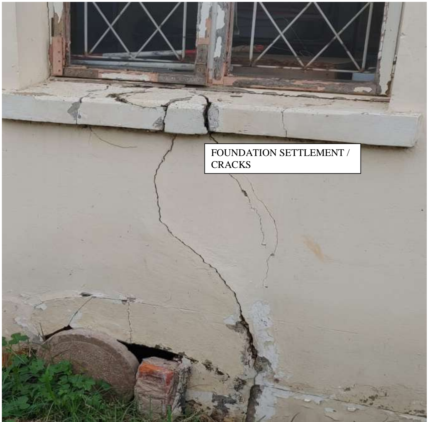
FIGURE 5 : SETTLEMENT OF FOUNDATION / CRACKS
