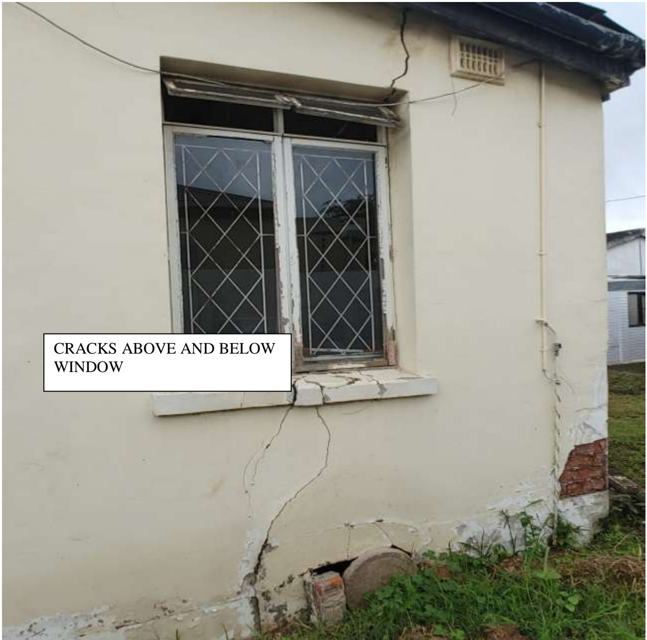
FIGURE 4 : SETTLEMENT OF FOUNDATION / CRACKS
