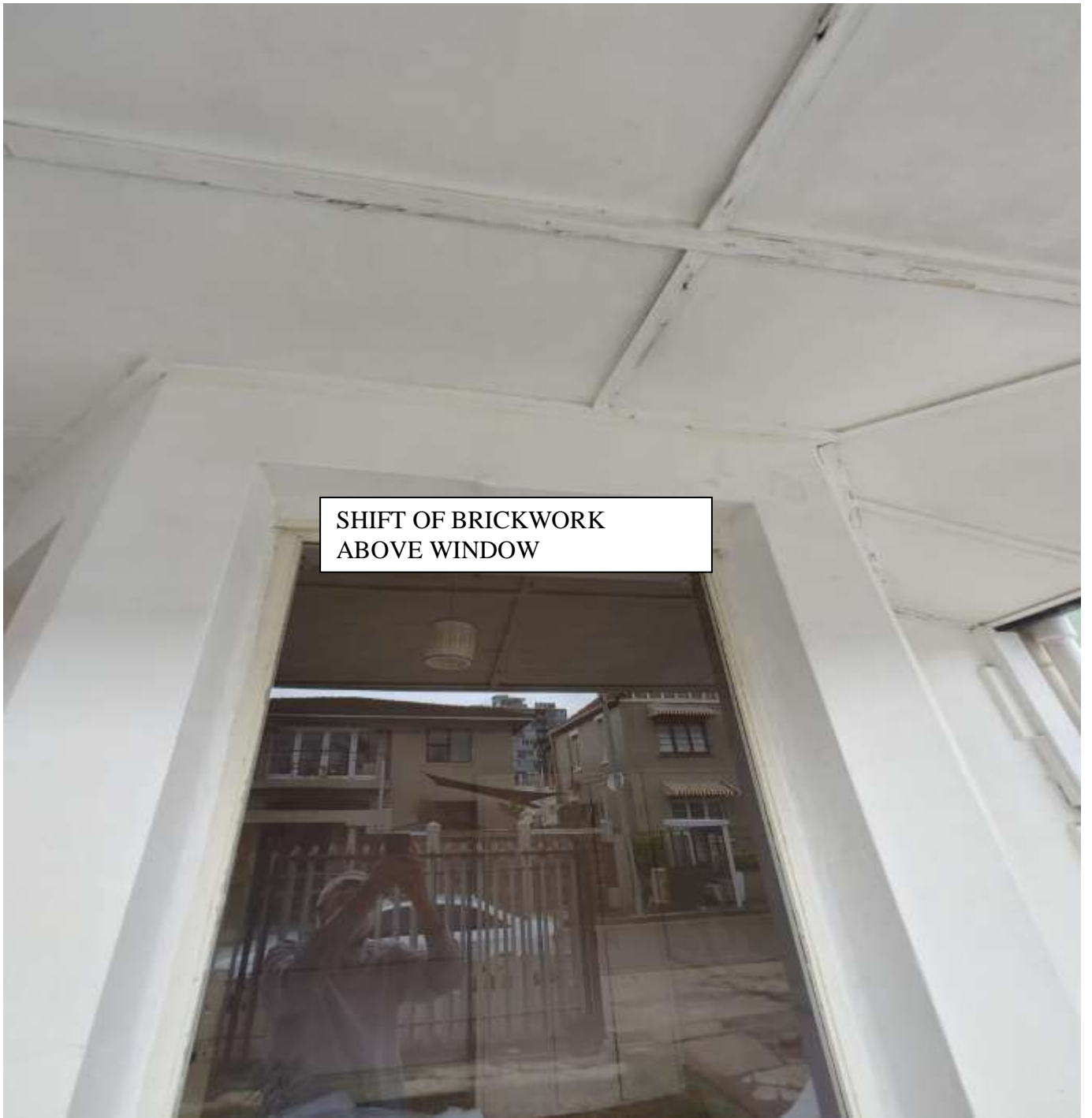
FIGURE 2 : SETTLEMENT OF HEADER COURSE
