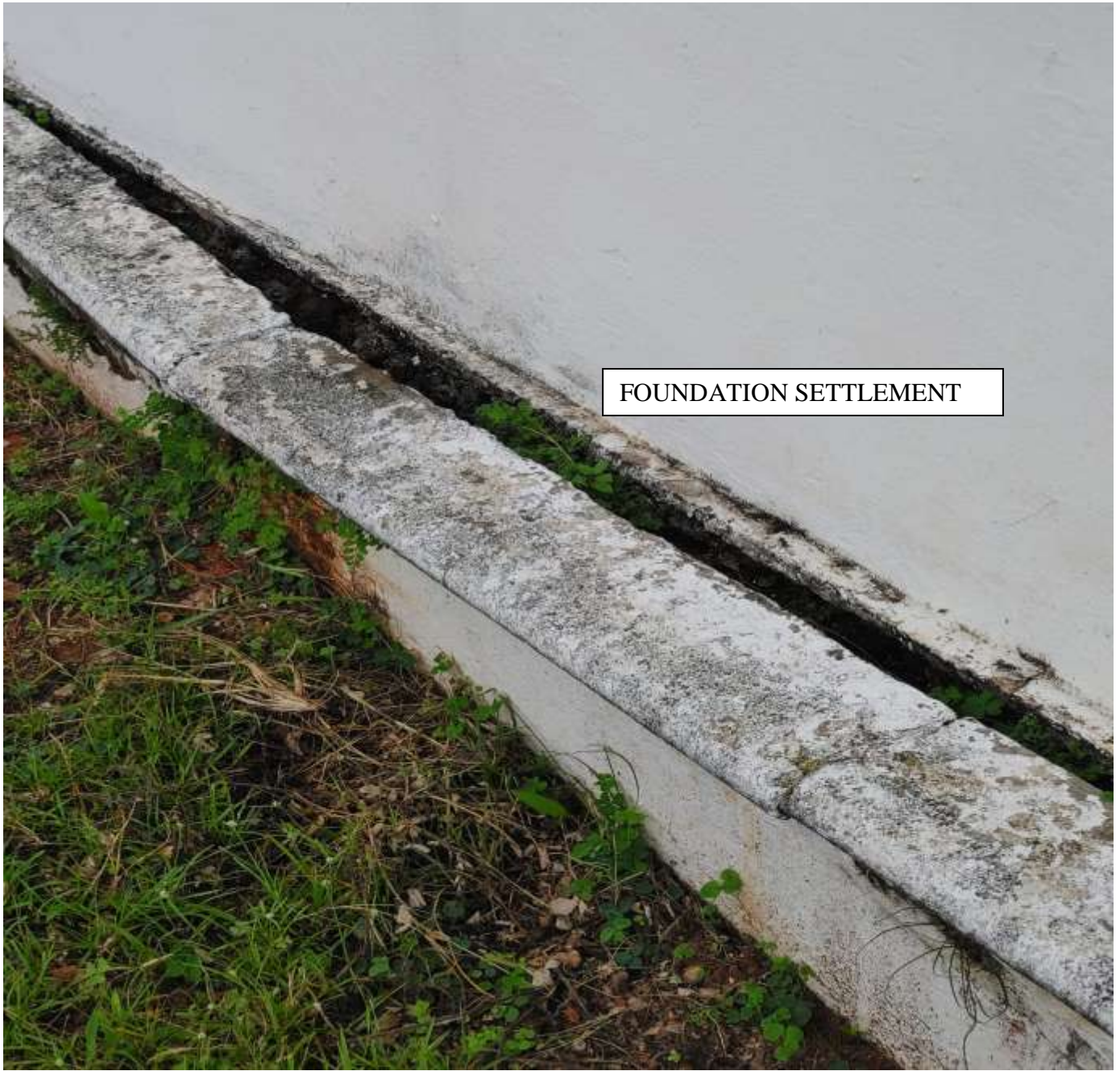
FIGURE 6 : SETTLEMENT OF FOUNDATION / CRACKS
