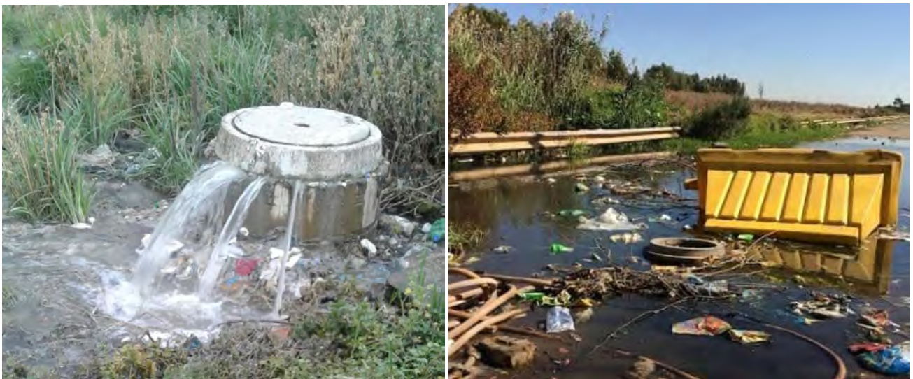
Figure 1-9: Lack of / poor maintenance of municipal services in the area of Riverlea which includes overflowing manholes and sewage pipes and poor waste collection services.
