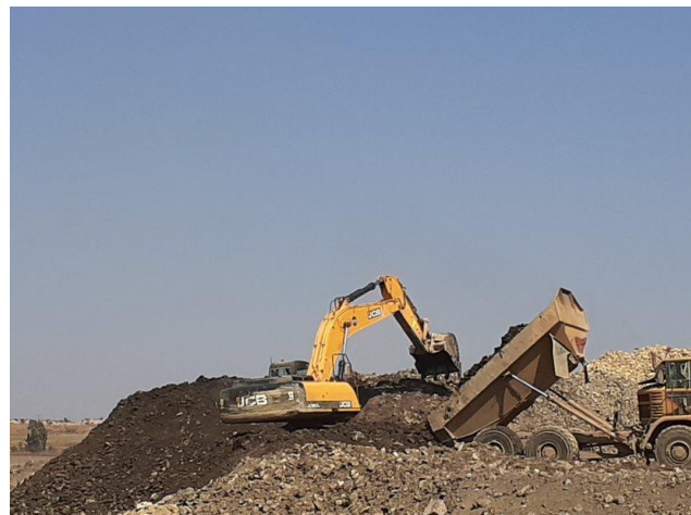
Example of newly removed silt being dumped by the ADT, and turned by a front-end loader
