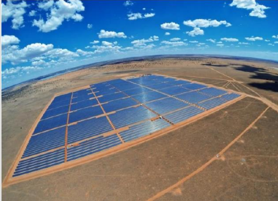
Figure 1.1: Photo showing a typical PV facility
