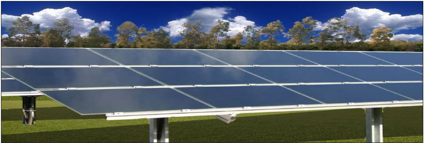
Figure 4. Frontal view of PV arrays mounted on fixed mounting systems
