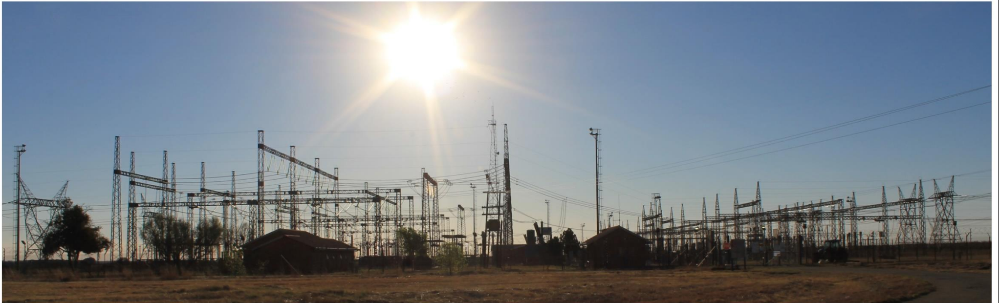
Theseus Main Transmission Station
