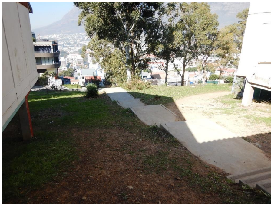
Figure 6A before: (Staircase 2) addition of steel handrails and balustrades on external stairs and walkways.
