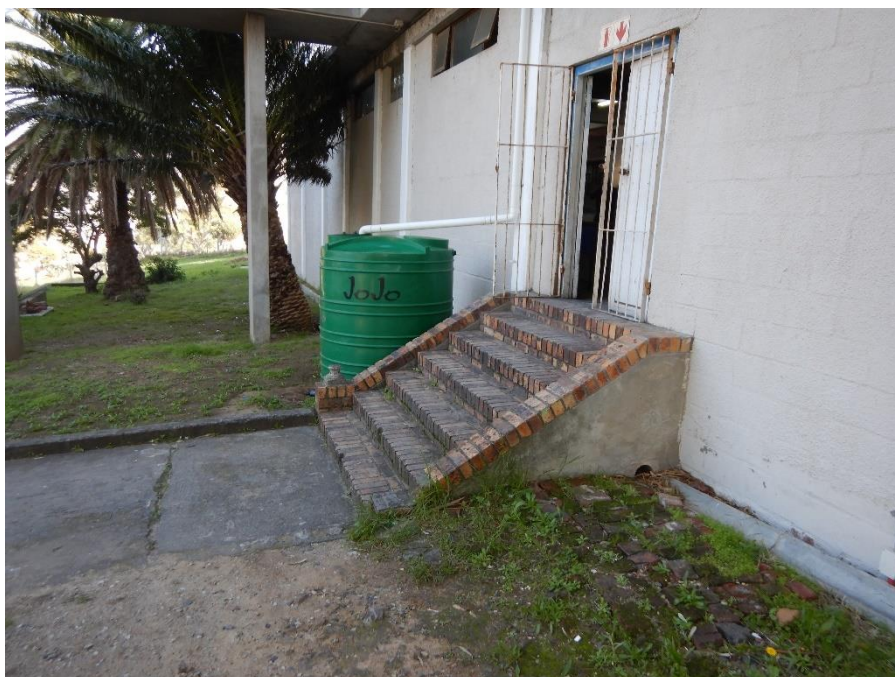
Figure 7A before: (Staircase 3) addition of steel handrails and balustrades on external stairs and walkways.
