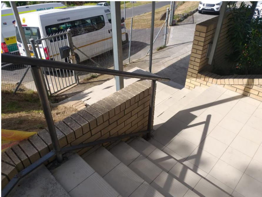
Figure 5A before: (Staircase 1) addition of steel handrails and balustrades on external stairs and walkways.
