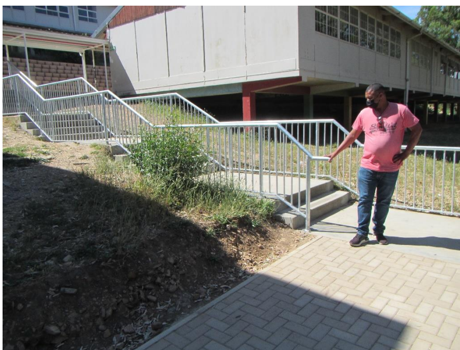
Figure 6B after: (Staircase 2) addition of steel handrails and balustrades on external stairs and walkways.
