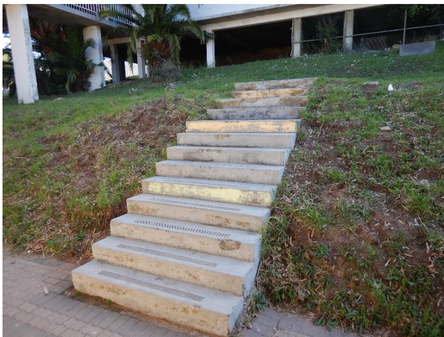
Figure 9A before: (Staircase 5) addition of steel handrails and balustrades on external stairs and walkways.
