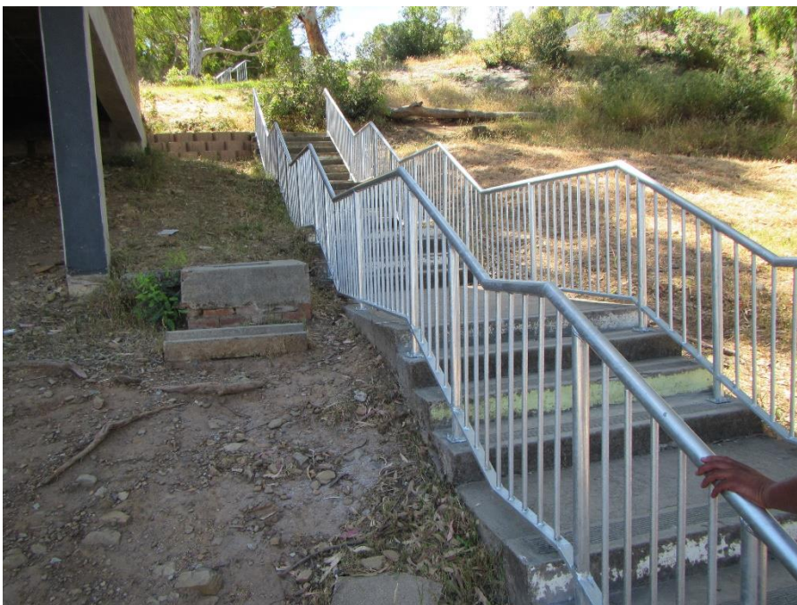
Figure 10B after: (Staircase 6) addition of steel handrails and balustrades on external stairs and walkways.
