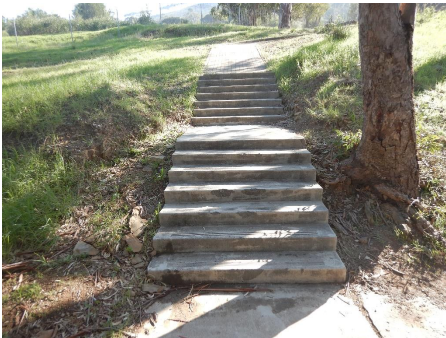
Figure 11A before: (Staircase 7) addition of steel handrails and balustrades on external stairs and walkways.
