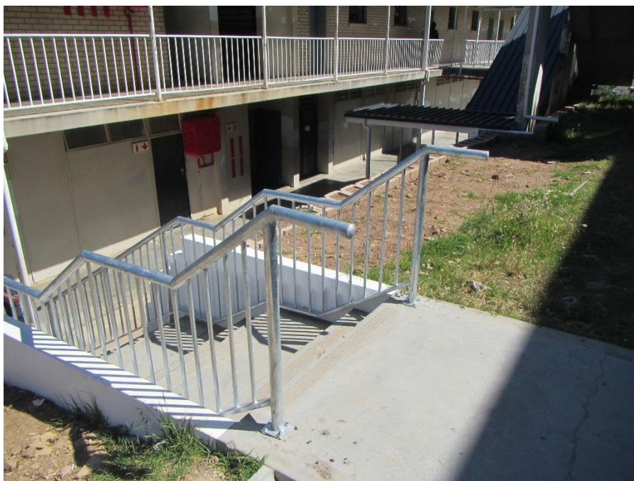
Figure 9B after: (Staircase 5) addition of steel handrails and balustrades on external stairs and walkways.
