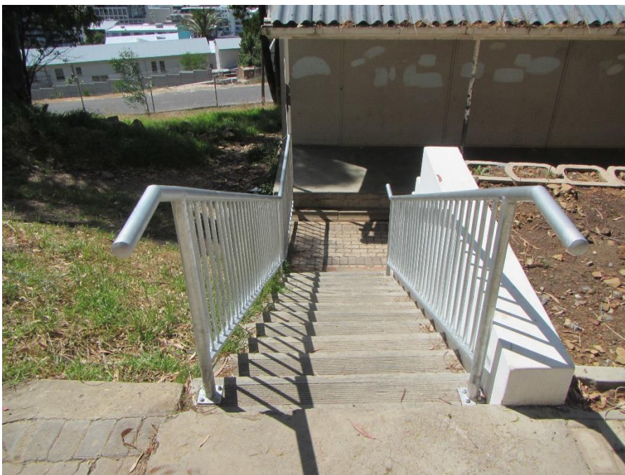
Figure 8B after: (Staircase 4) addition of steel handrails and balustrades on external stairs and walkways.
