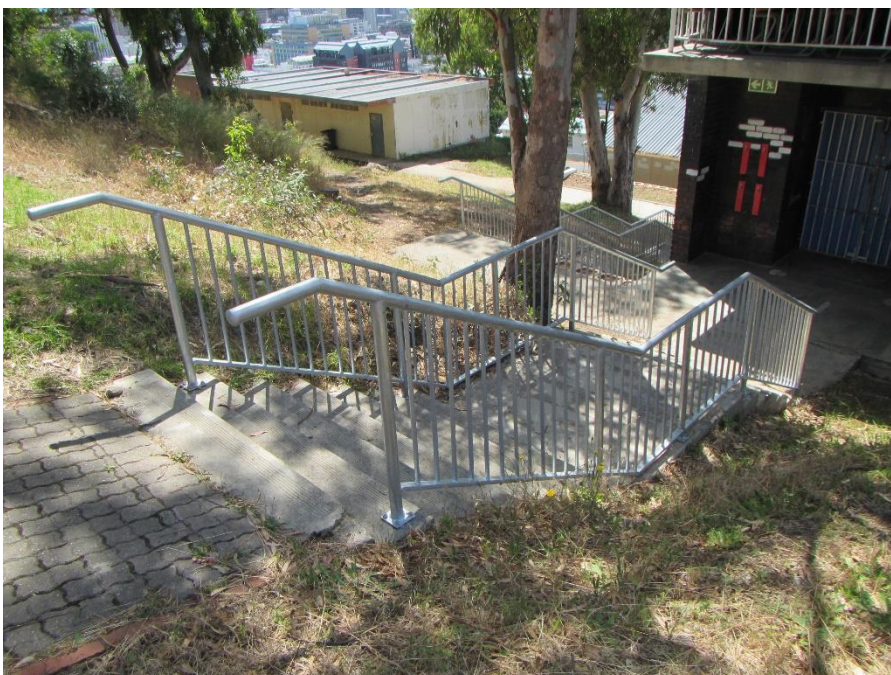
Figure 11B after: (Staircase 7) addition of steel handrails and balustrades on external stairs and walkways.
