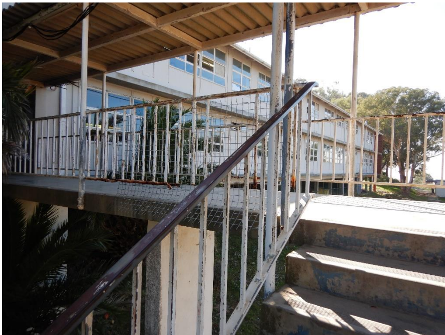
Figure 15A before: Corroded handrails and balustrades.
