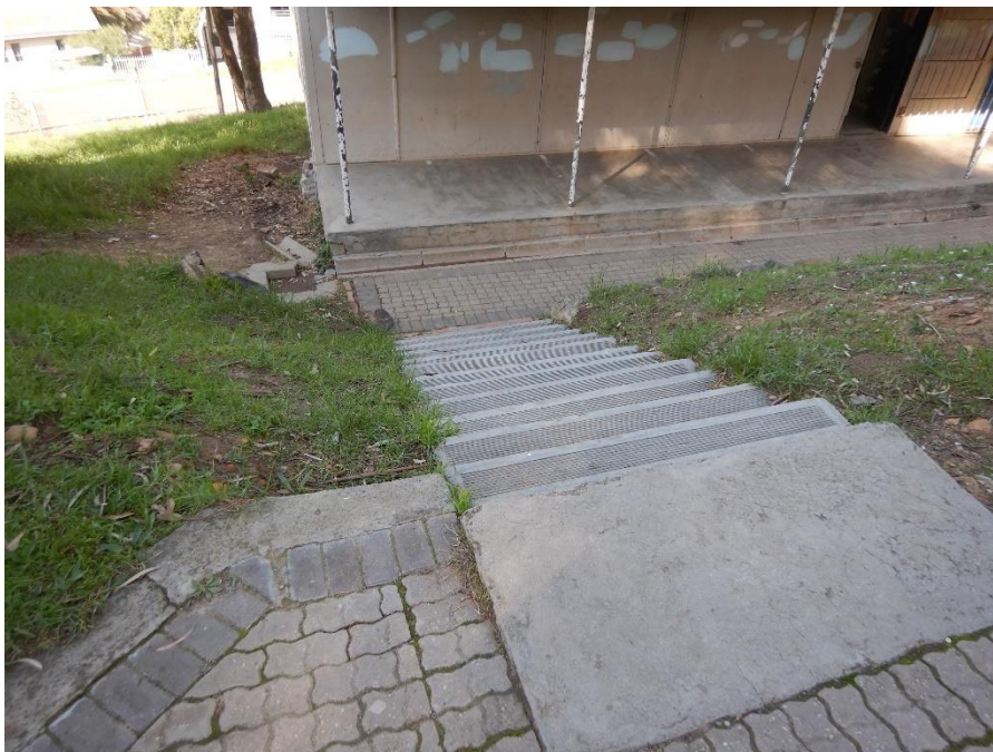
Figure 8A before: (Staircase 4) addition of steel handrails and balustrades on external stairs and walkways.
