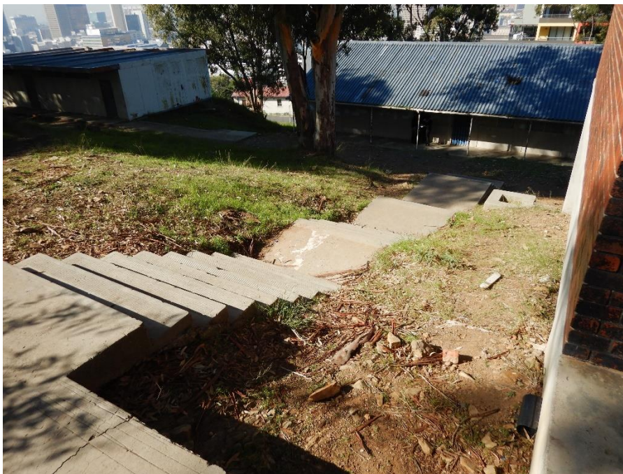
Figure 10A before: (Staircase 6) addition of steel handrails and balustrades on external stairs and walkways.
