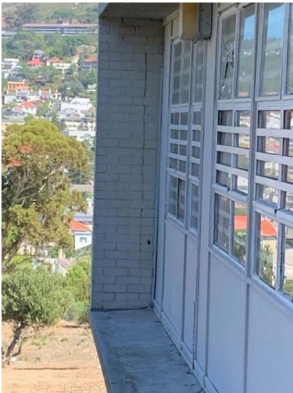
Figure 4.17: cracking in structural brickwork.
