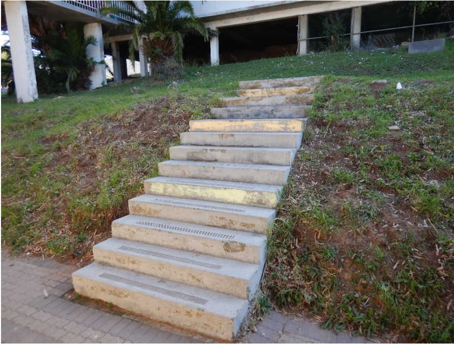
Figure 4.10: Staircase 5 (see site plan) – to receive safety handrails on both sides.
