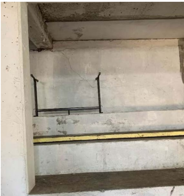
Figure 4.19: concrete spalling and cracking.
