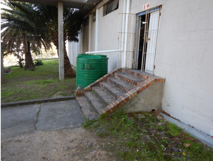
Figure 4.8: Staircase 3 (see site plan) – to receive safety handrails on both sides.
