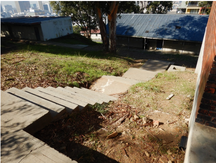
Figure 4.11: Staircase 6 (see site plan) – to receive safety handrails on both sides.
