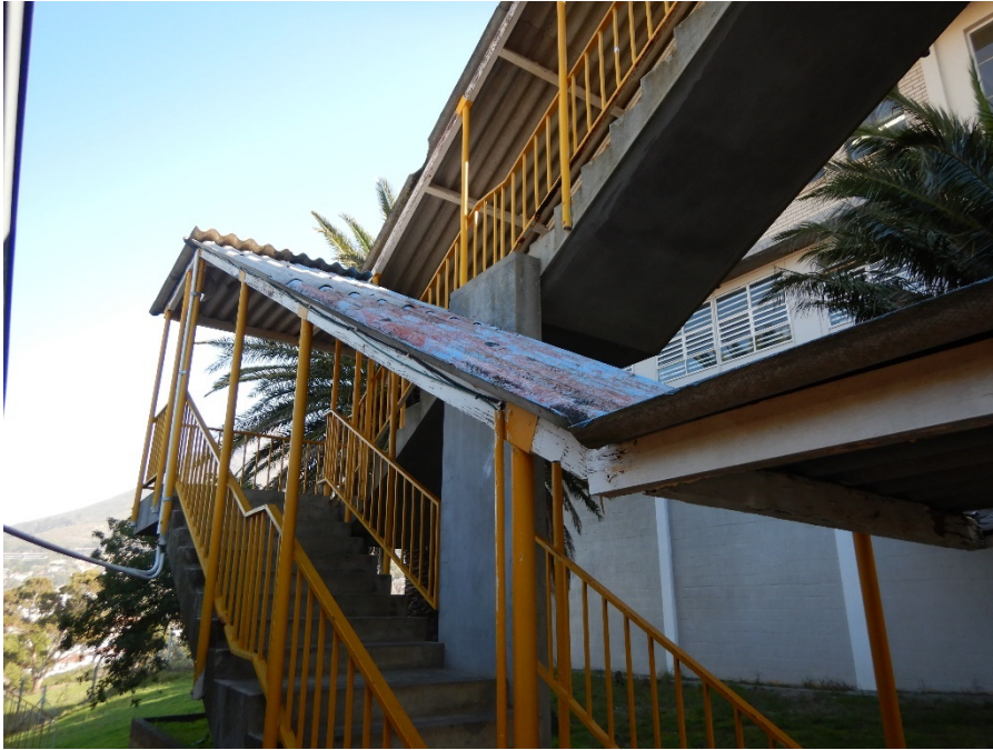
Figure 4.2: Condition of roof canopy 2 - asbestos sheeting unstable, unfit for school use.
