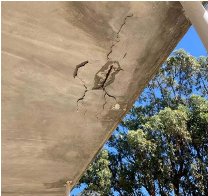
Figure 4.18: concrete spalling and cracking.
