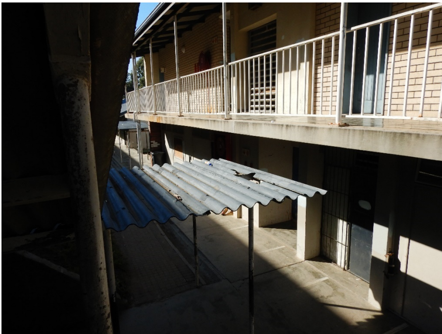
Figure 4.3: Condition of roof canopy – holes causing hazardous conditions for learners.
