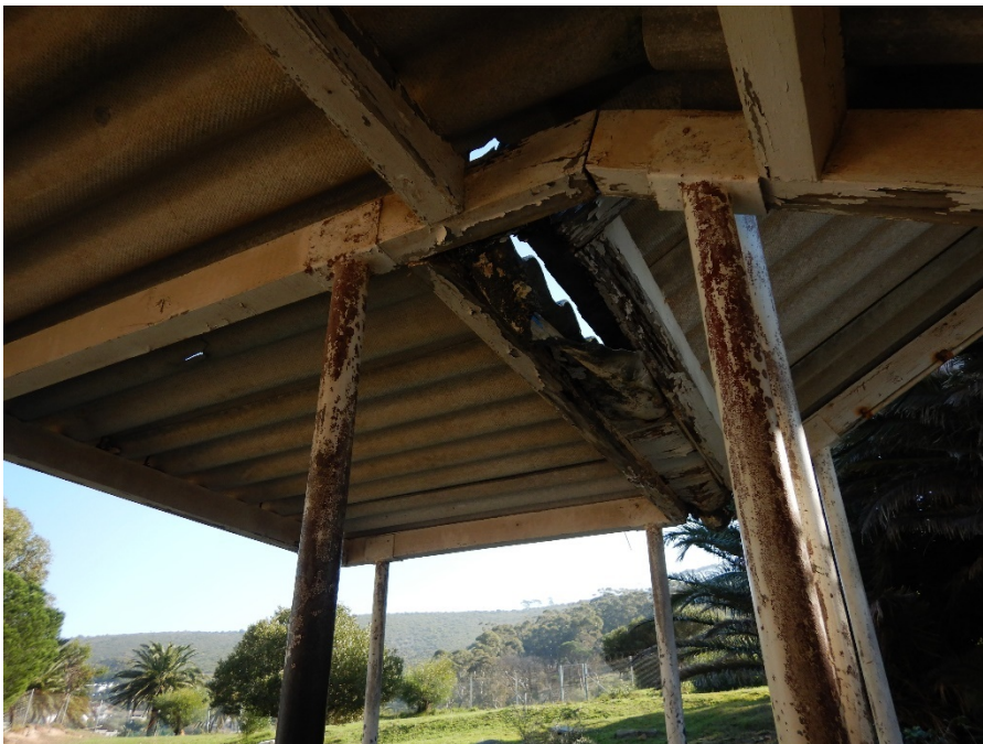
Figure 4.5: Condition of roof canopy – exposed rusted fixing members hazardous for learners.
