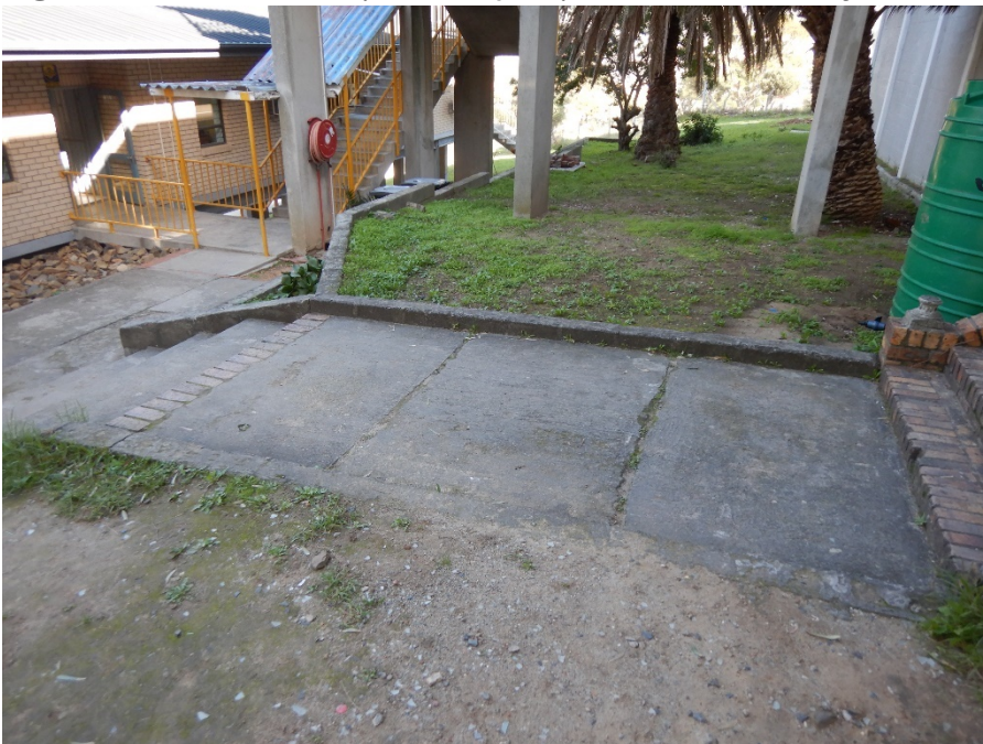
Figure 4.7: Staircase 3 (see site plan) – to receive safety handrails on both sides.
