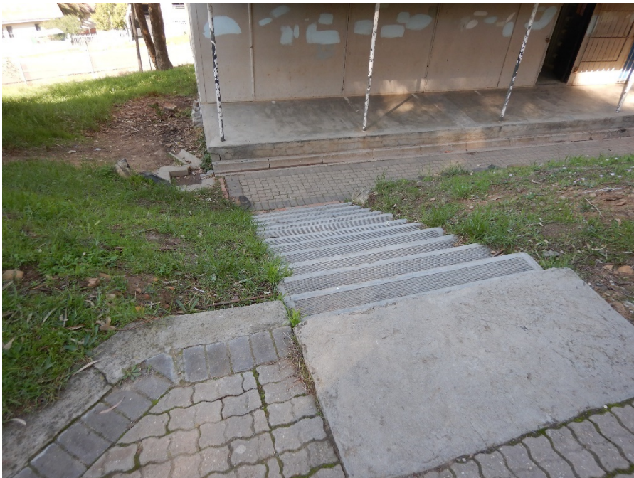
Figure 4.9: Staircase 4 (see site plan) – to receive safety handrails on both sides.
