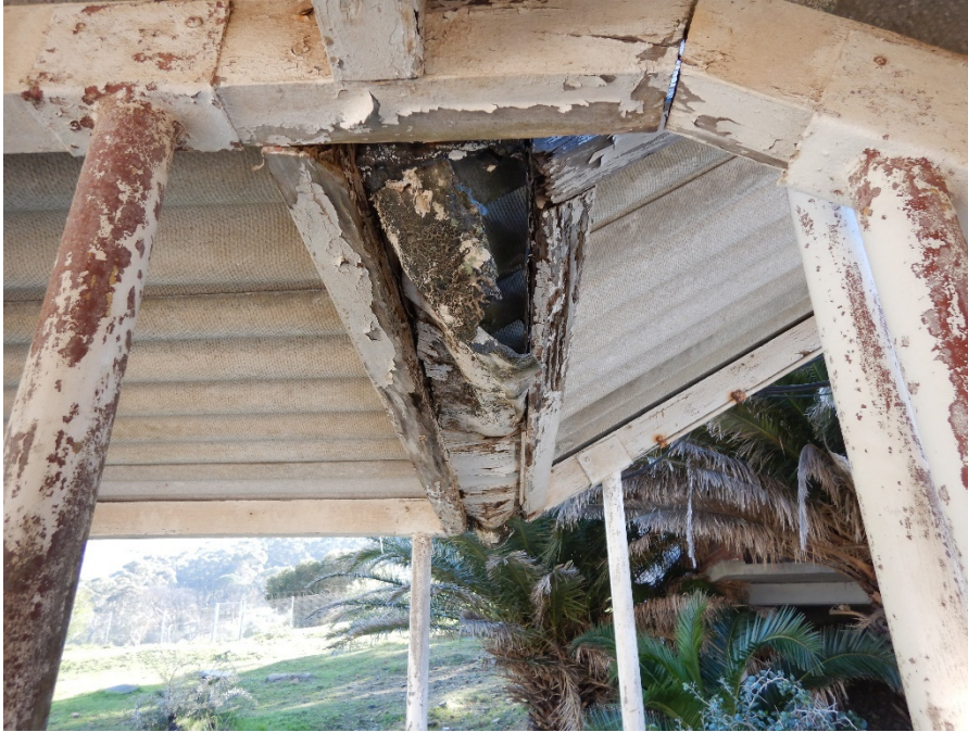
Figure 4.4: Condition of roof canopy – rotting of timber members impacting structural integrity.
