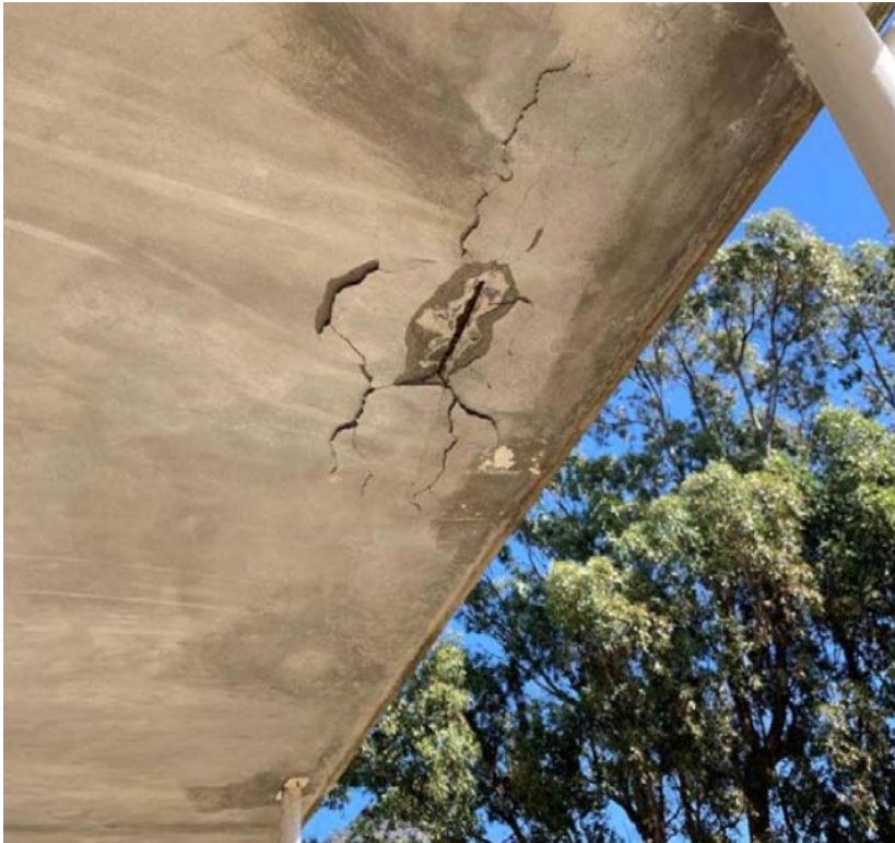
Figure 4.18: concrete spalling and cracking.
