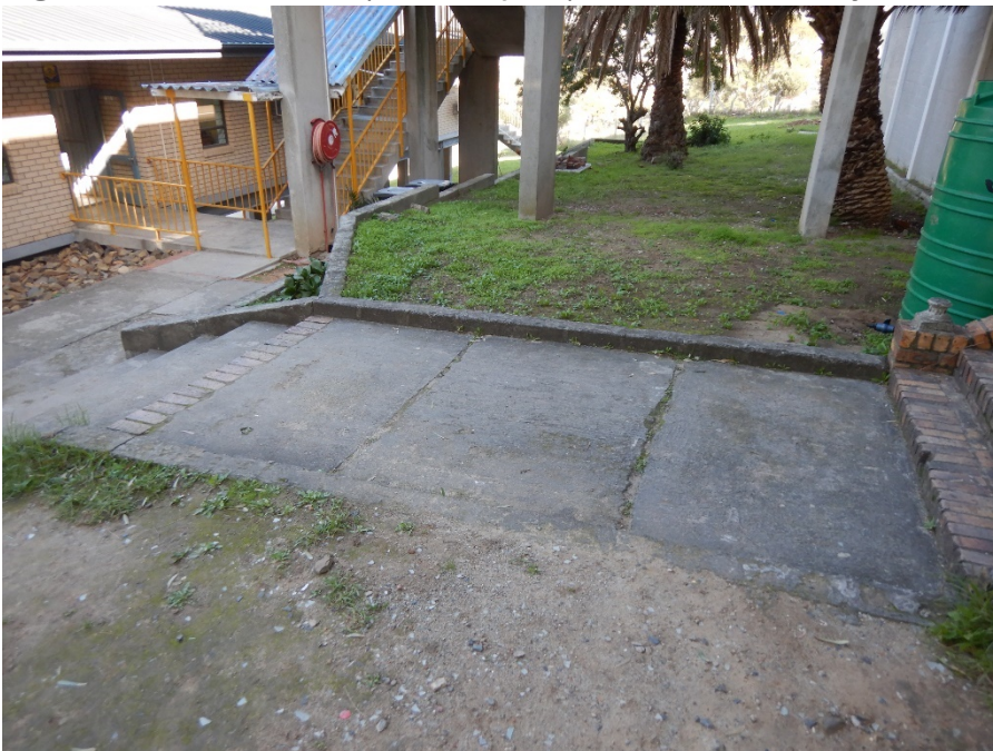
Figure 4.7: Staircase 3 (see site plan) – to receive safety balustrades on both sides.
