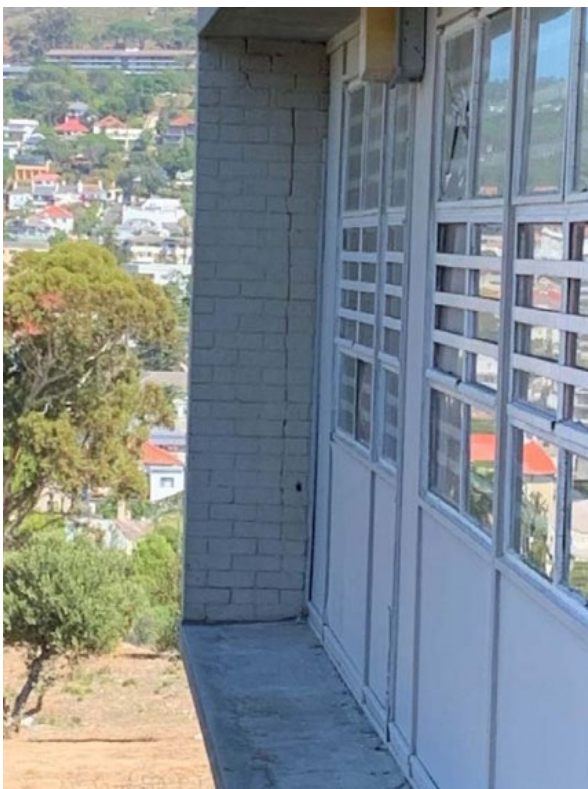
Figure 4.17: cracking in structural brickwork.
