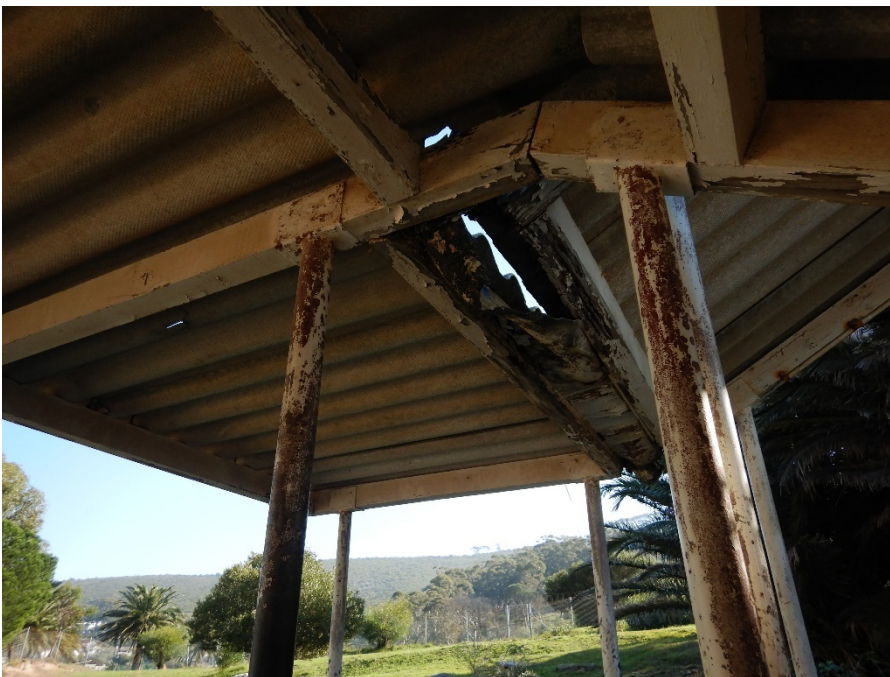
Figure 4.5: Condition of roof canopy – exposed rusted fixing members hazardous for learners.
