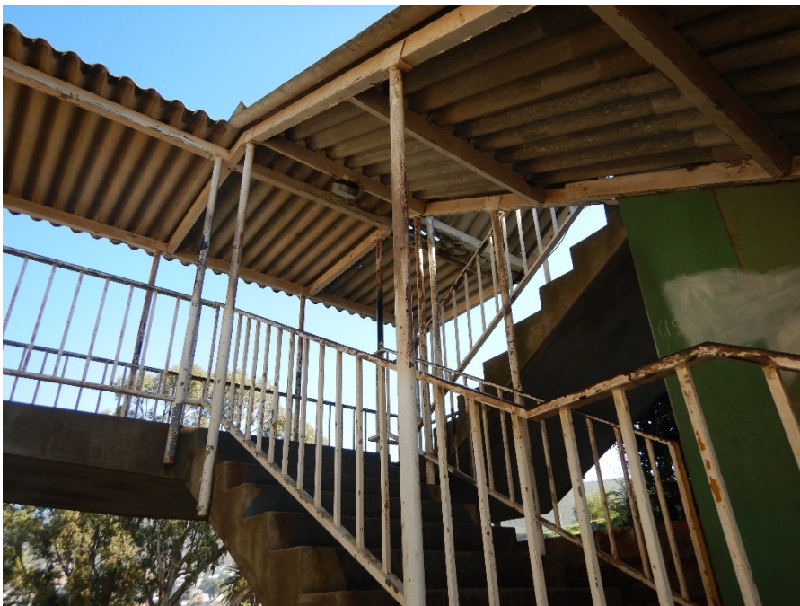
Figure 4.1: Condition of roof canopy – steel posts weathered and corroded.
