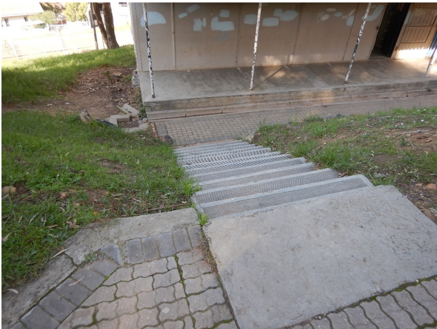
Figure 4.9: Staircase 4 (see site plan) – to receive safety balustrades on both sides.
