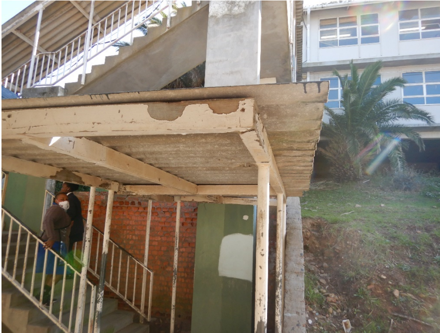
Figure 4: Condition of roof canopy – asbestos sheeting to be replaced.
