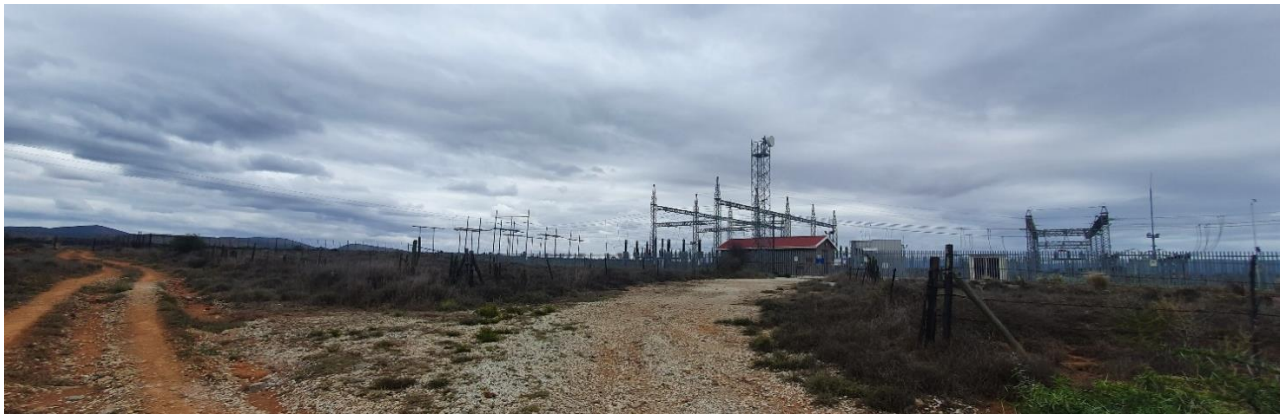
Figure 5-6: Existing Skilpad Substation located on the south-eastern portion of the property
