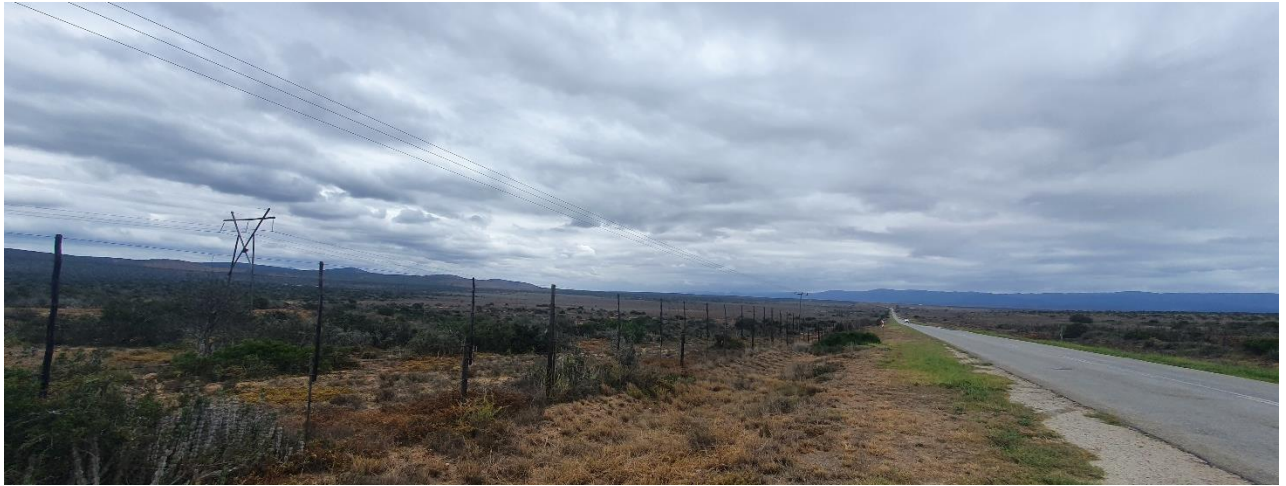
Figure 5-9: Powerlines routed adjacent to the R75
