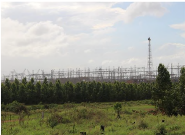
Plate 3 - Sub-station & Communication Tower
