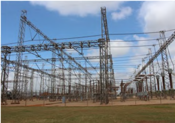
Plate 1 - Sub-station Bus Bars maximum height 10-15m
