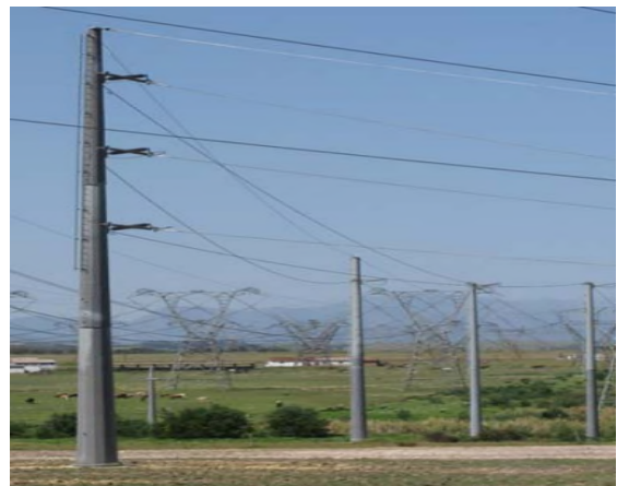
Plate 4 - 23-28m high, 132kV self-sustaining steel monopole tower.
