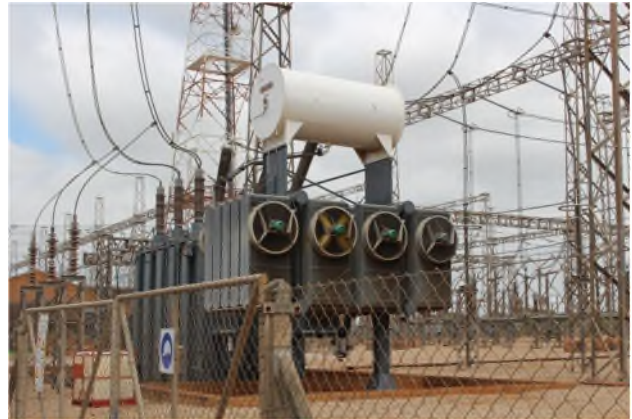
Plate 2 - Transformer with oil storage tank above.
