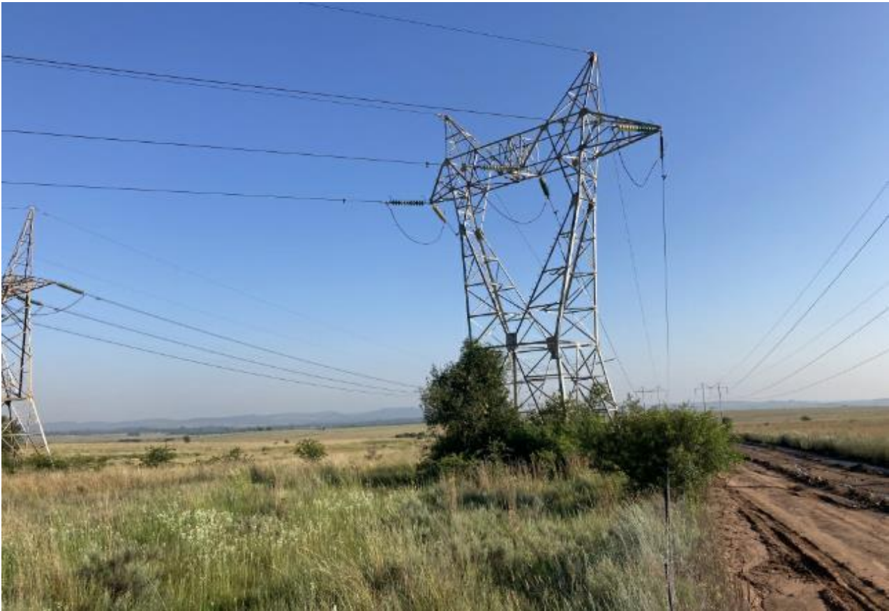
Figure 8: High voltage lines
