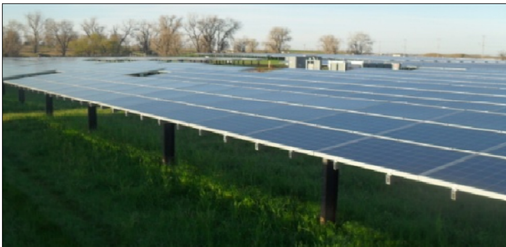
Figure 7: Frontal views of the PV arrays mounted on 1-axis horizontal tracker
