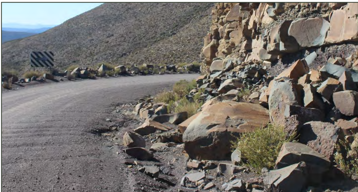
Figure 11: Falling rocks at Komsberg Pass
