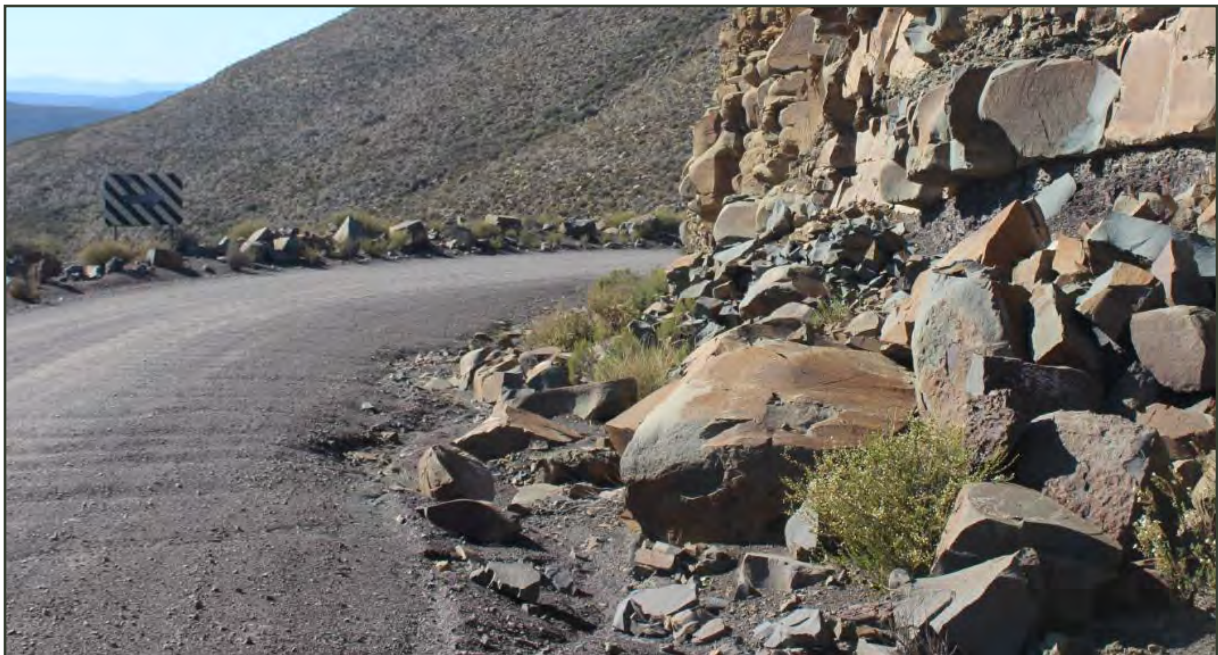
Figure 11: Falling rocks at Komsberg Pass
