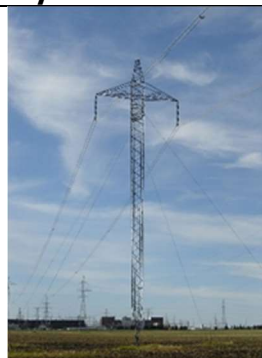
Plate 6-3: Free standing metal lattice towers.
