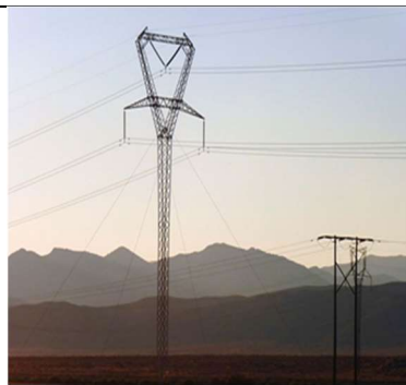
Plate 6-2: Guy line supported steel structures.
