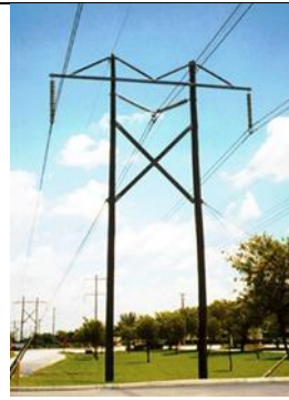
Plate 6-4: Multi-pole structures such as H-towers or K-towers.
