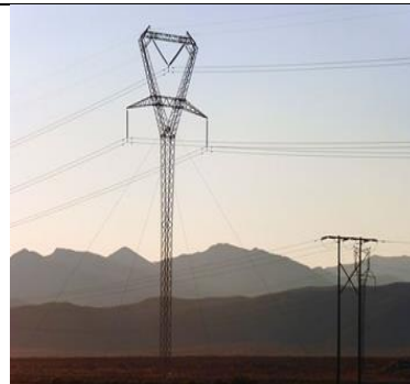
Plate 6-2: Guy line supported steel structures.
