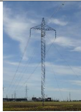
Plate 6-3: Freestanding metal lattice towers.
