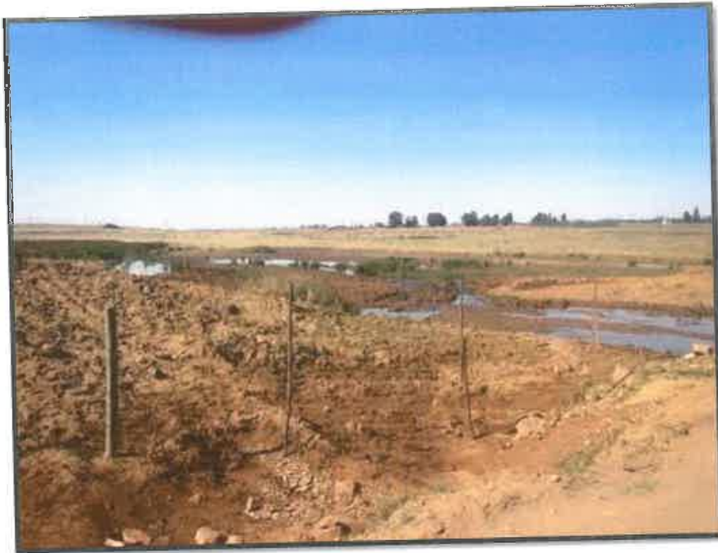
Photograph 7.1-16: The road works by the Mpumalanga Provincial Government Department of Public Works, Roads and Transport in Nkangala have created an unpleasant sight in the impeding of the wetland with the disposal of soil and rubble on the edges of the as wetland.
