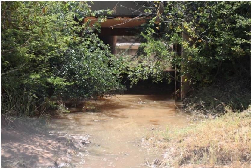
Figure 20: (Left) Culvert of Streamcrossing No. 3 at the site. Water visible in picture gathered after substantial rains (RF. Terblanche, 2019)
