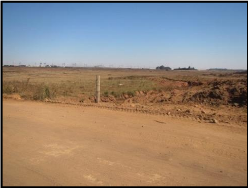
Photograph 9.1-15: The road works have created a visual intrusion and impeding on the wetland with the disposal of soil and rubble on the edges of the as wetland (north east side) (26° 02' 097" S; 0,28° 53' 027" E).
