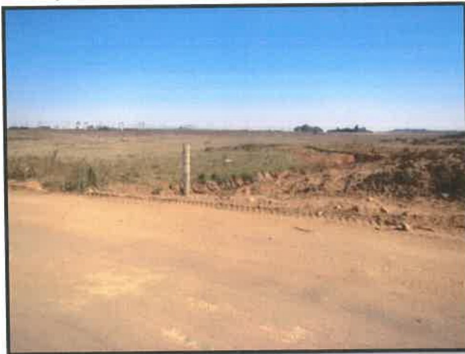
Photograph 9.1-15: The road works have created a visual intrusion and impeding on the wetland with the disposal of soil and rubble on the edges of the as wetland (north east side) ( 26^{\circ} 02' 097'' S; 0,28^{\circ} 53' 027'' E).
