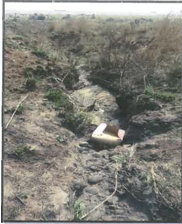
Figure 14: The drainage continues from the colbet into the sensitive area near the Arbor Siding operation area.
