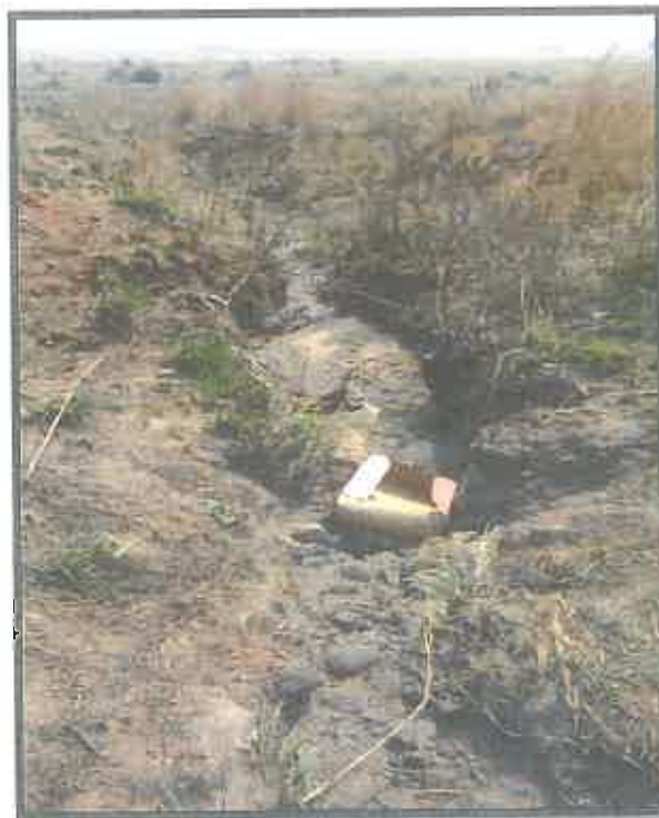
Figure 14: The drainage continues from the colbet into the sensitive area near the Arbor Siding operation area.
