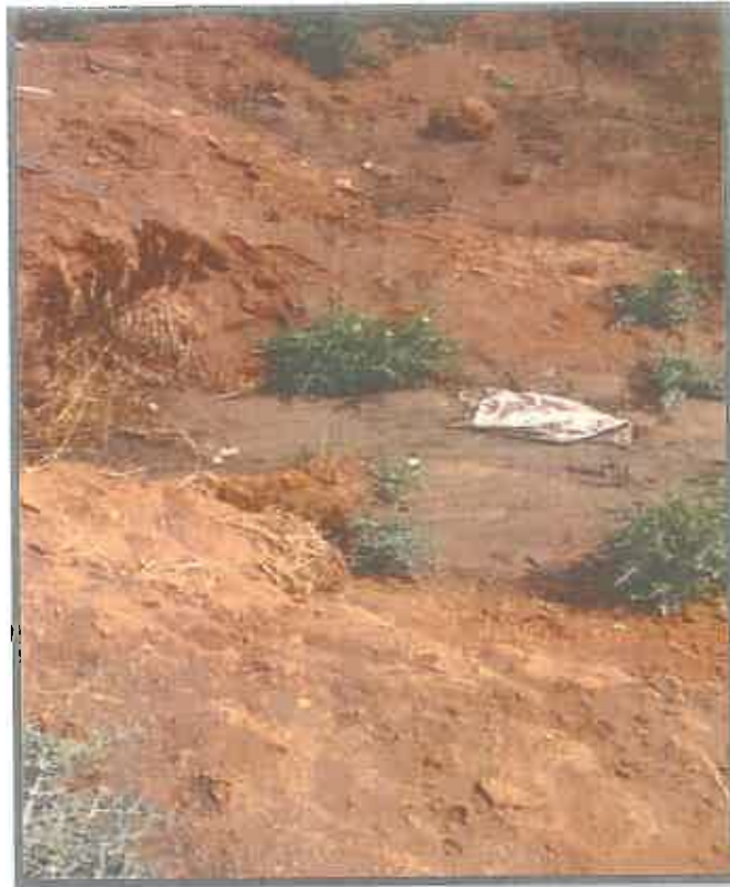
Figure 13: Stormwater colbet from R555 used to drain stormwater.
