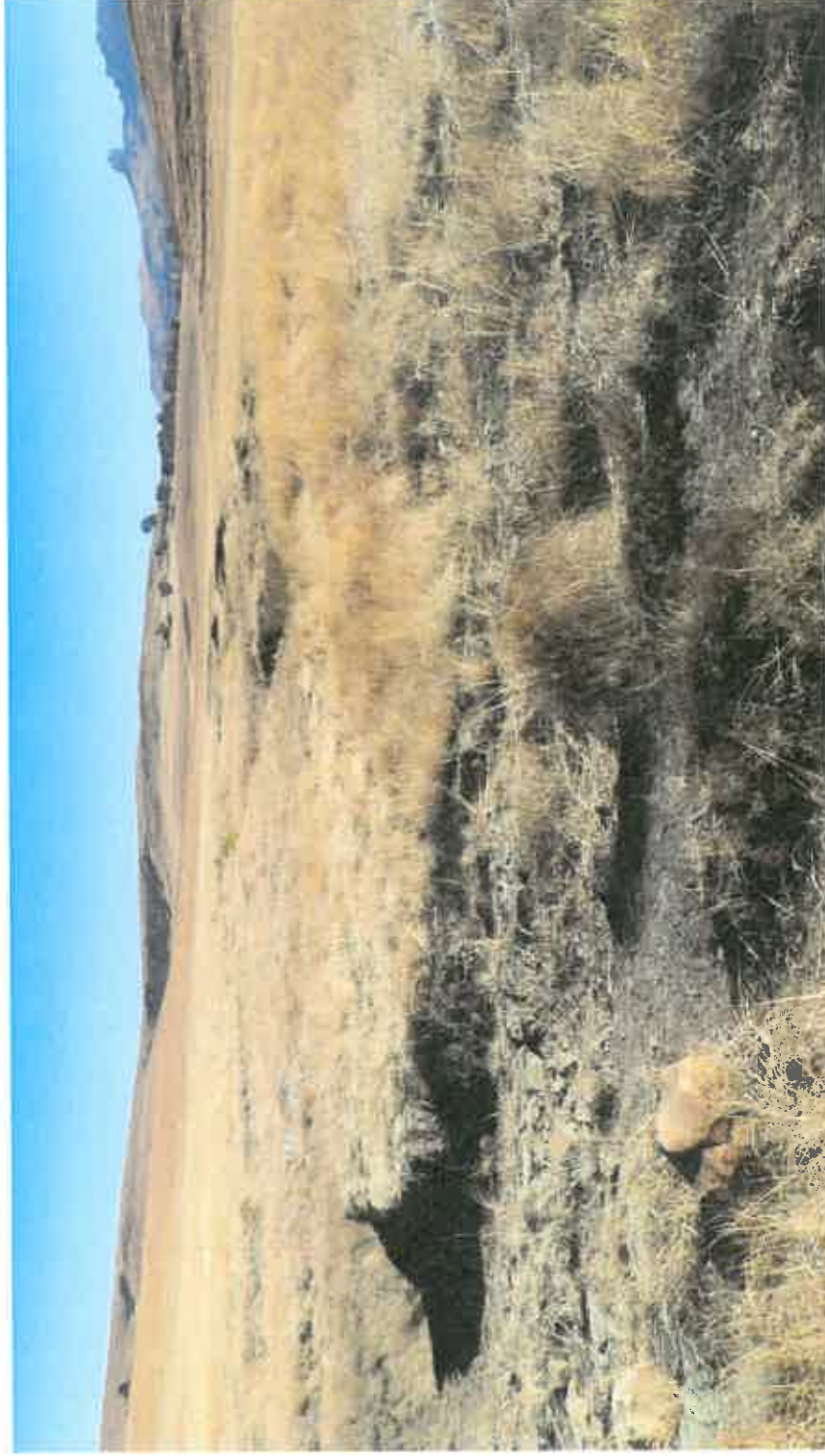
Figure 13: Example of a stream crossing (severe erosion) with poorly constructed road – needs rehabilitation.
