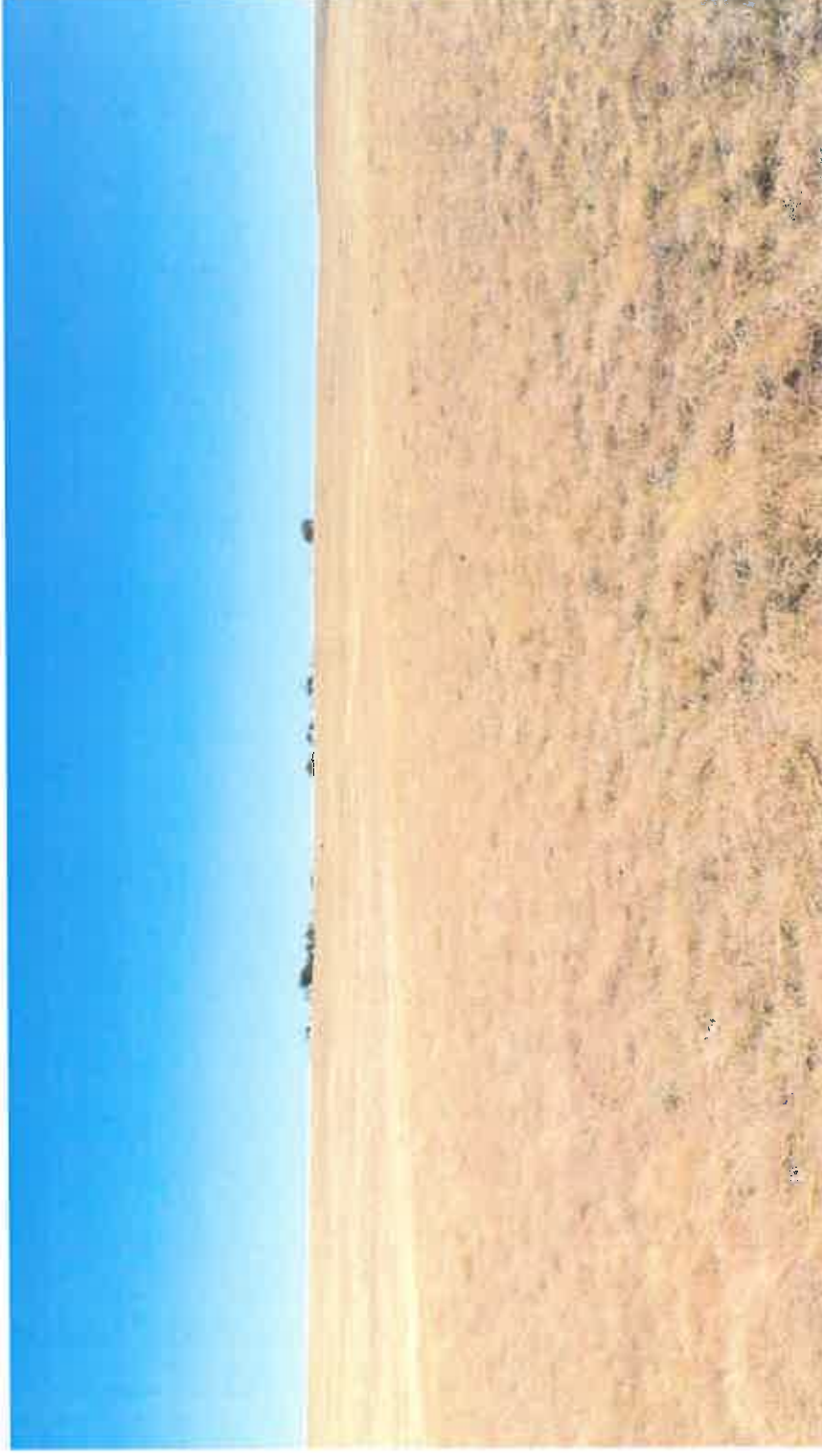
Figure 10: The condition of the basal layer in a fair condition.
