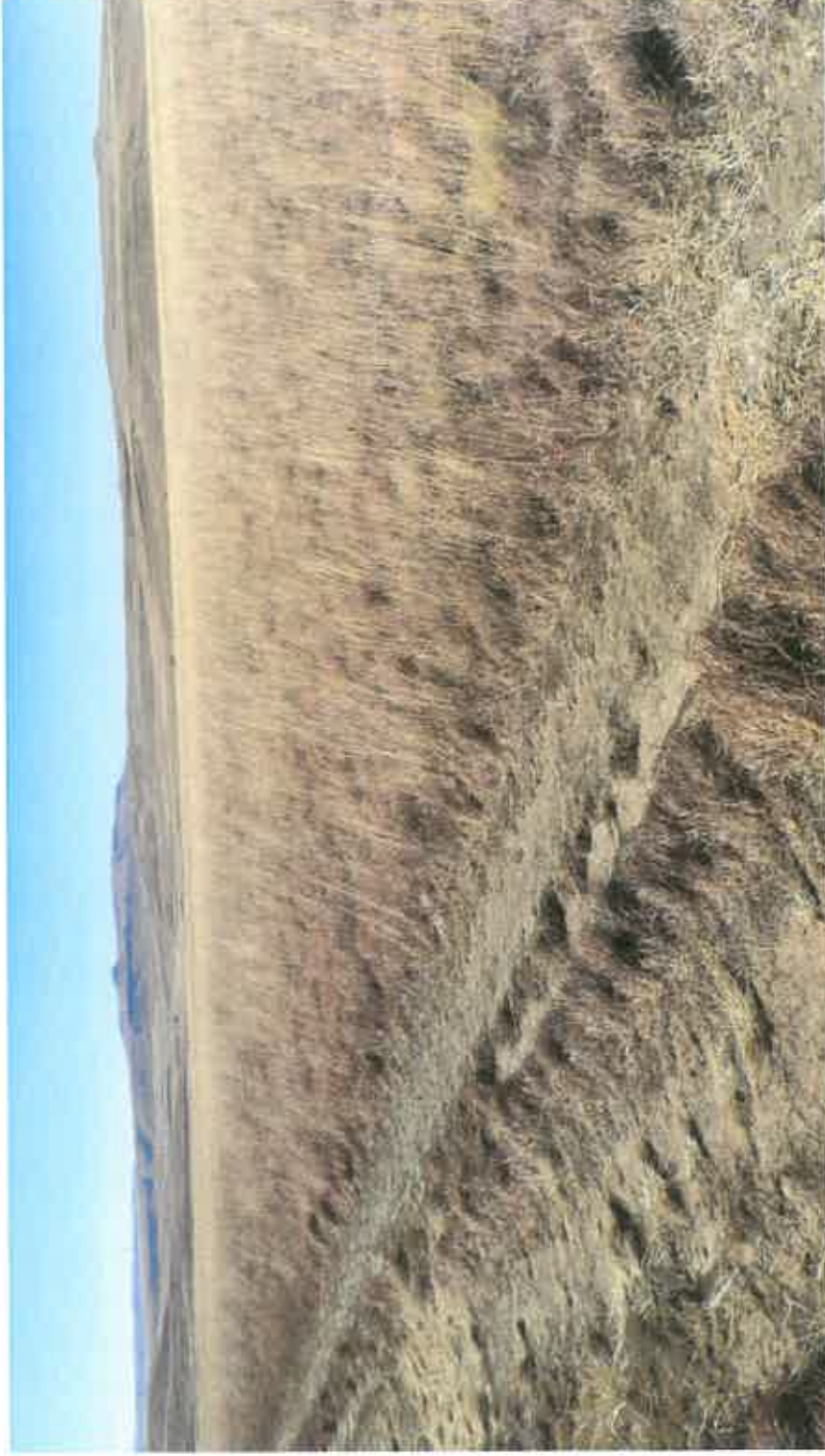
Figure 20: Although the road is on a flat section of the property, early signs of erosion present – it will be important to include the maintenance of the road as part of the future management strategy.
