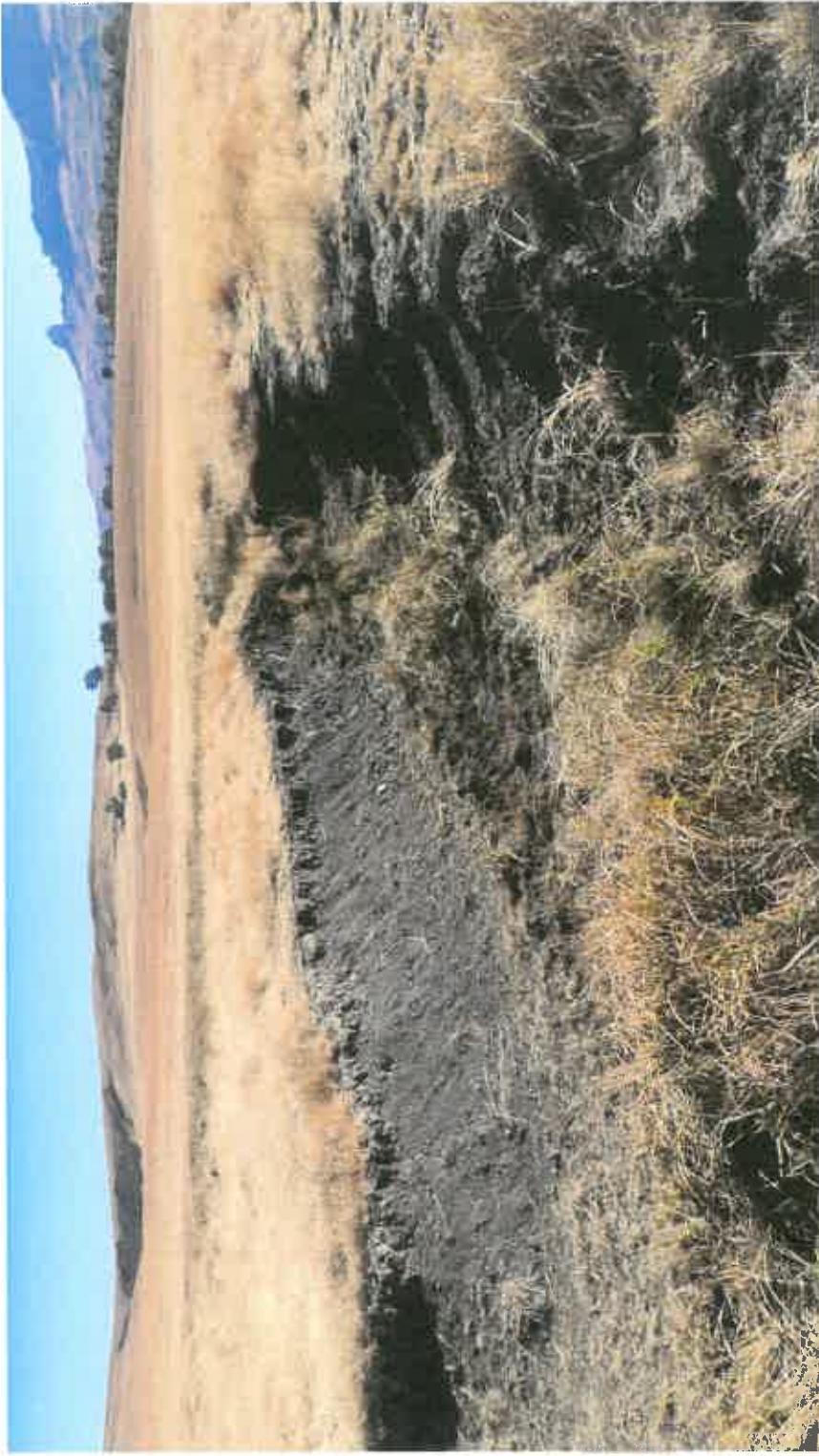
Figure 17: Modified drainage channel with accelerated erosion – rehabilitation recommended.
