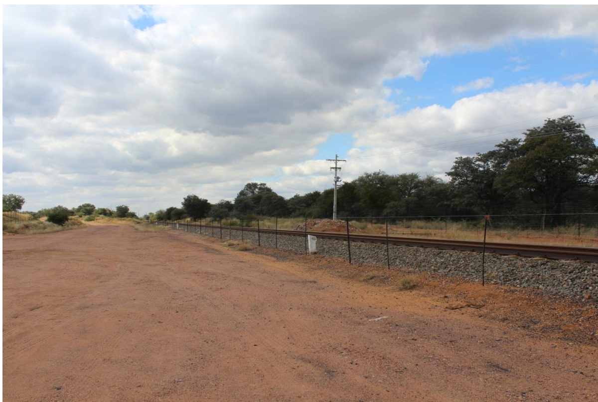
Figure 3: View of the existing railway track (right) and cleared servitude (left) for the completion of Boikarabelo 36km rail link
