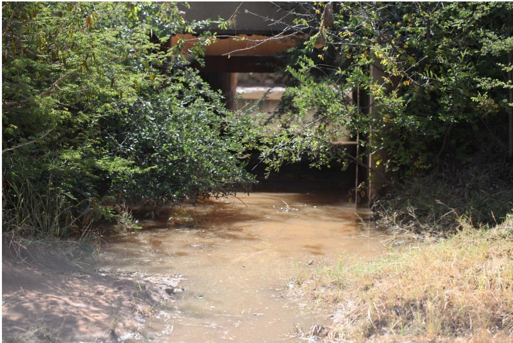
Culvert underneath railway line at Streamcrossing No3 at the site. Water visible in picture gathered after substantial rains.
