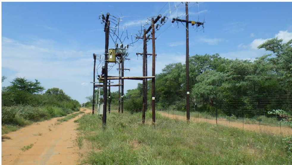
Figure 20: At KOP10 the existing infrastructure supplying electricity to the farms are visible near the fence, but it is effectively screened by the vegetation when one move into the veld.
