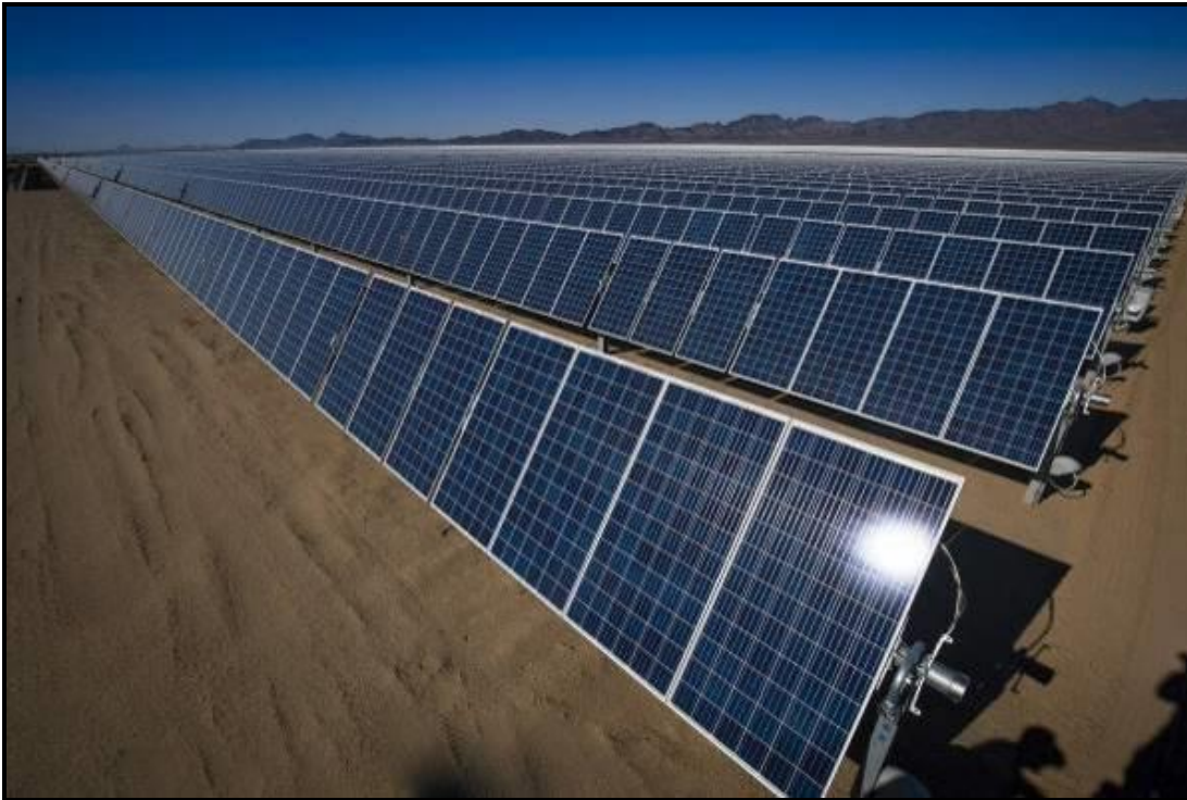
Photograph 1.1: Typical PV SEF facility
