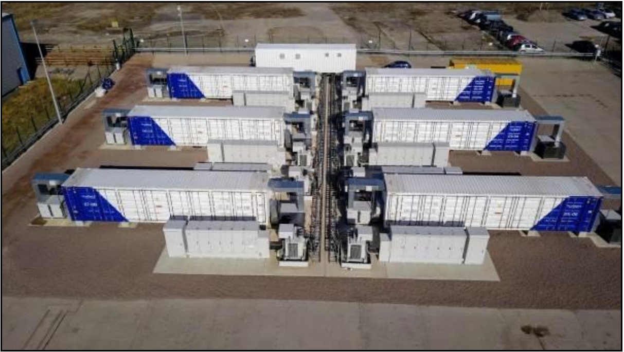
Photograph 1.2: Example of BESS located in storage containers
