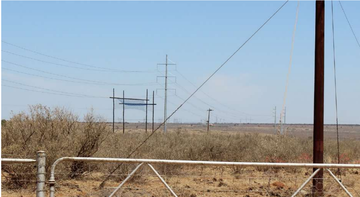
Figure 1-22 Electrical infrastructure as seen from Photo Site VNW017. The Mookodi Substation can be seen in the background.
