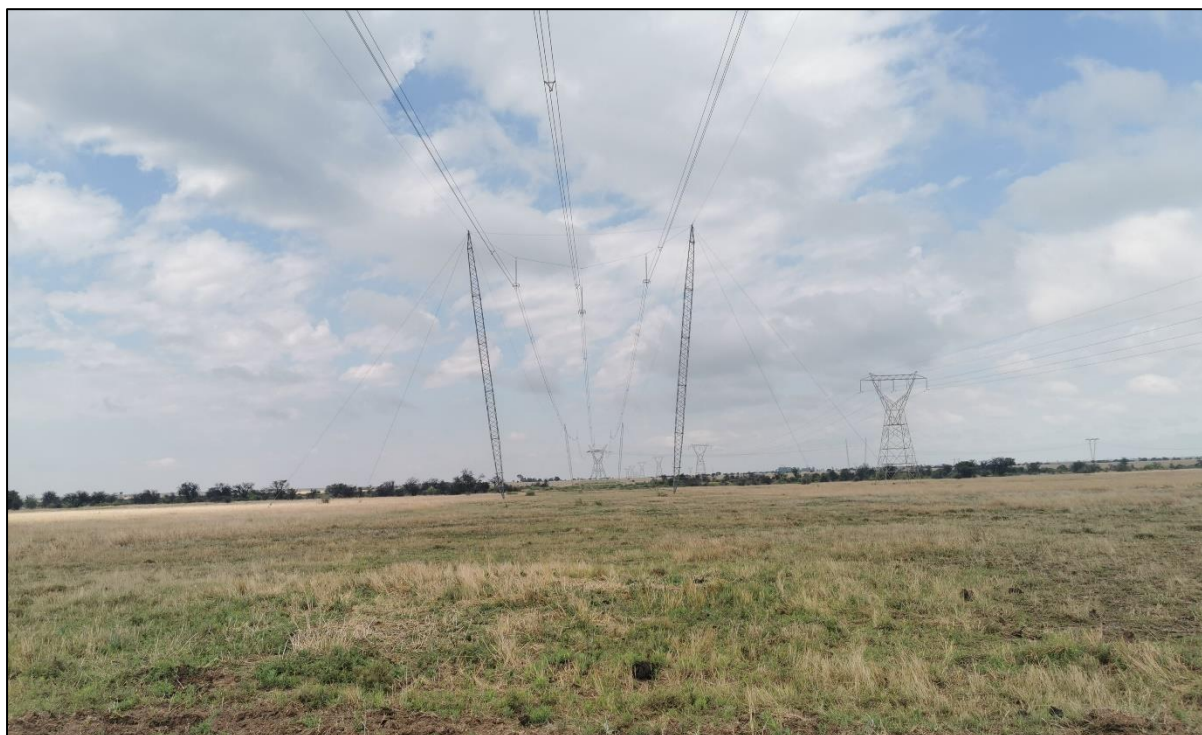
Figure 9-1: Existing powerline servitude in the AoI (October 2022)
