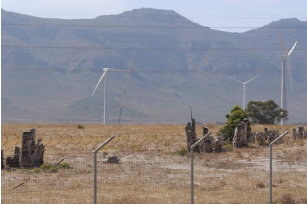
Plate 19, Gouda Wind Farm, turbines being erected with the use of a crane.
