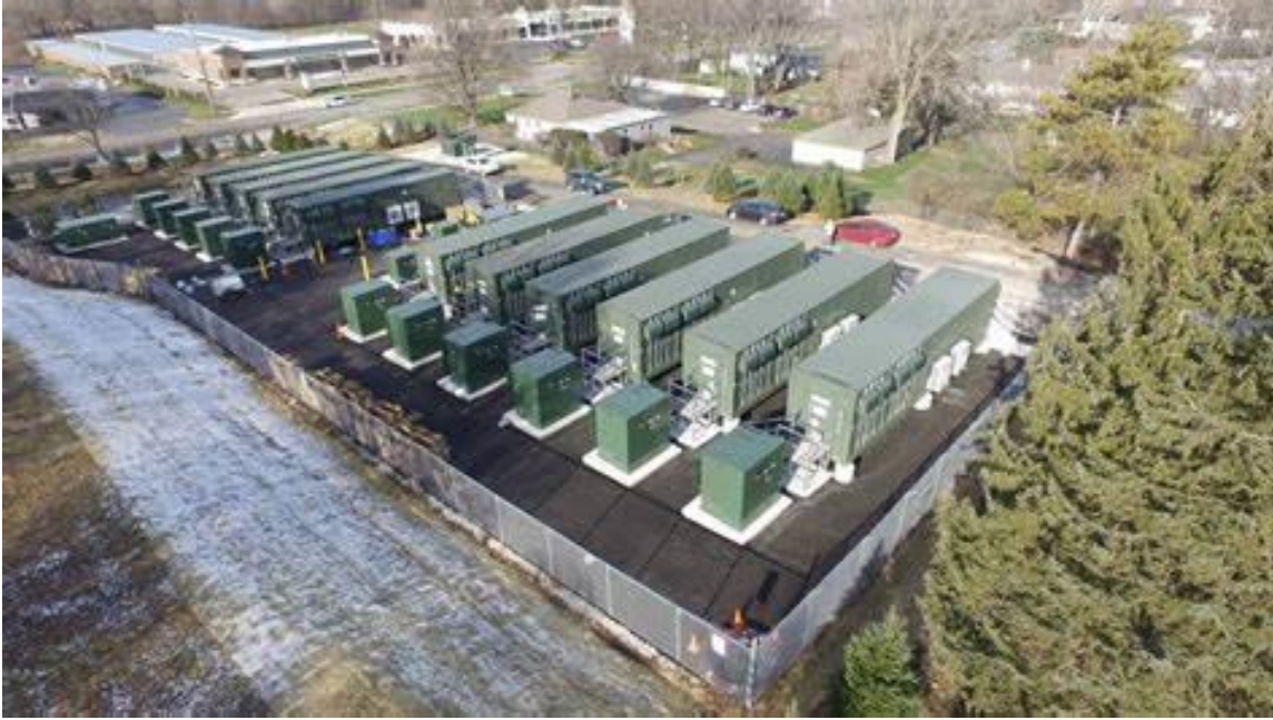
PLATE 1 TYPICAL BATTERY ENERGY STORAGE SYSTEM
