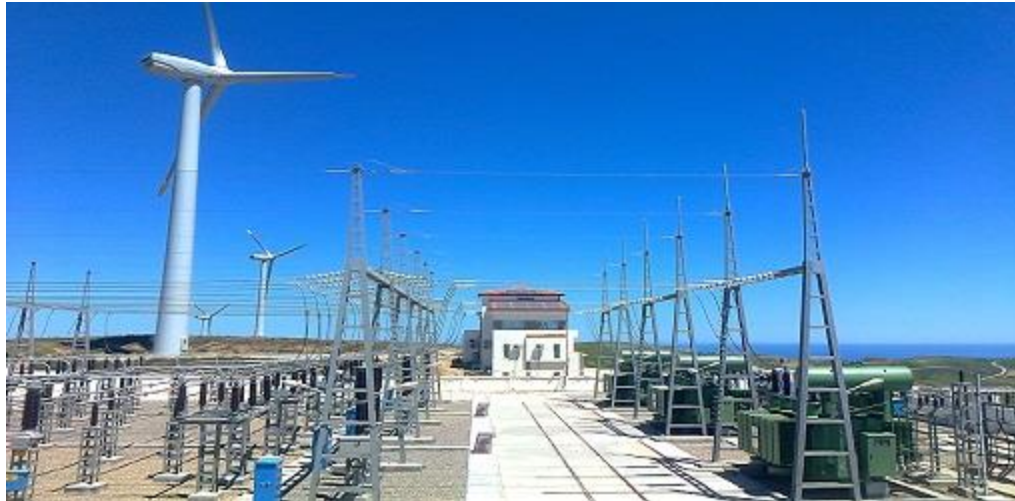
PLATE 2, BUS BARS ARE THE HIGHEST SUBSTATION ELEMENTS IN PICTURE
