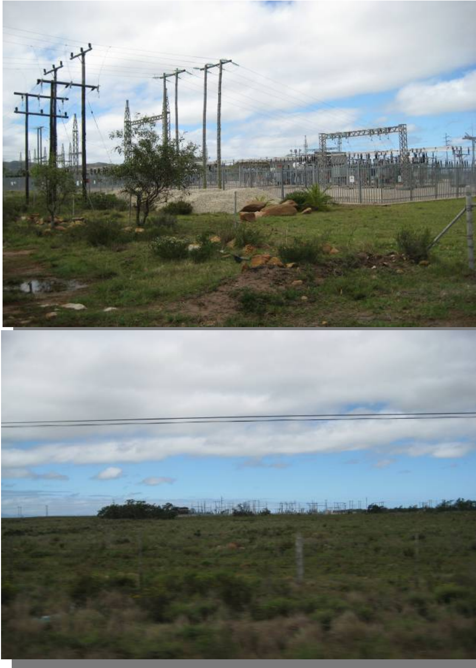
Figure 3.1: Melkhoutbosch substation, near the N2-R330 interchange north of Humansdorp
